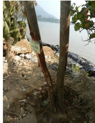
Photo 12 – Mechanical injuries were observed on the trunks of the retained trees E68.
