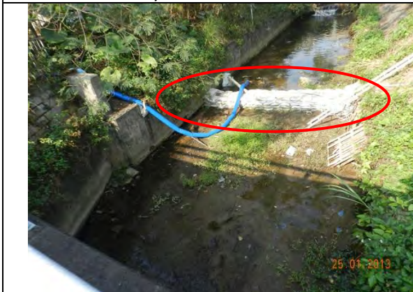
Photo 15 – Wai Ha river was blocked by sand bags to fragment a works area. The running water of the river was pumped to the end of the works area and then released back to the river.
