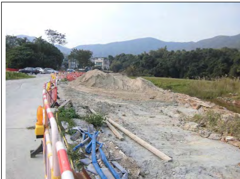
Photo 1: An uncovered sand stockpile was observed, the Contractor should cover it with tarpaulin sheet to prevent fugitive dust during dry season.
