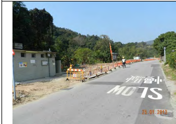
Photo 3 – Temporary hoardings have been erected along the west of Tung Tsz Road near the refuse collection point.
