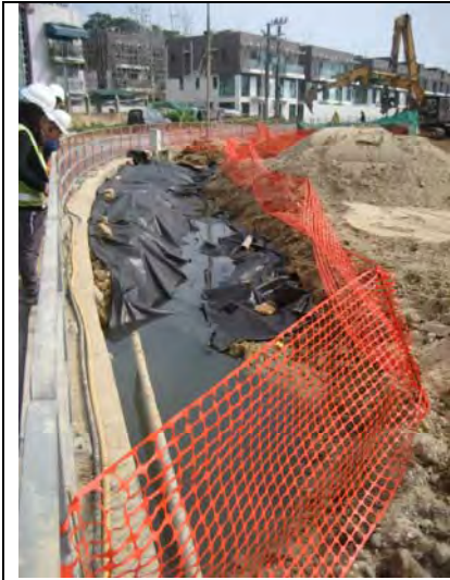
Photo 1: The exposed slope has been covered by tarpaulin sheet.
