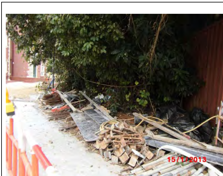
Photo 1: Scattered of construction waste was observed, the Contractor should improve housekeeping of the site.
