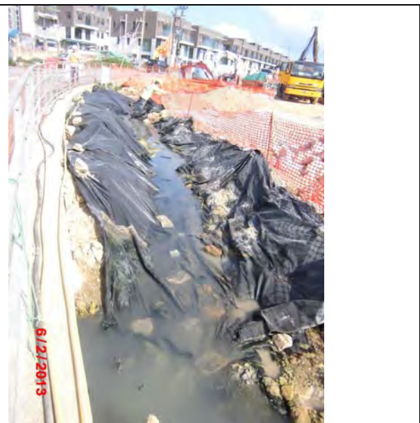
Photo 2: The channel for discharging water diversion should be improved.
