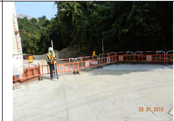
Photo 4 – Temporary hoardings have been erected on the path near Treasure Spot Garden II.
