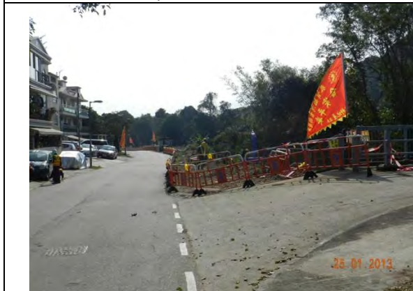
Photo 5 – New temporary hoardings have been erected at the northwest part of Tung Tsz Road near the removed tree group of T069-070.
