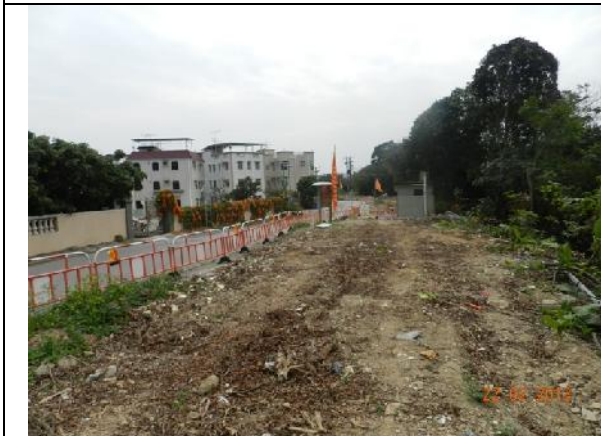
Photo 3 – Temporary hoardings have been erected along the west of Tung Tsz Road near the refuse collection point.
