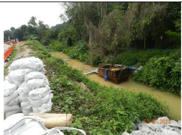
Photo 14 – The running water of the river was pumped to a sedimentation tank at the end of the works area. The filtrate was then discharged to the river with several sections of granules for further sedimentation.
