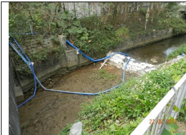
Photo 13 – Wai Ha River was blocked by sand bags to separate the works area. The running water of the river was pumped to the end of the works area.
