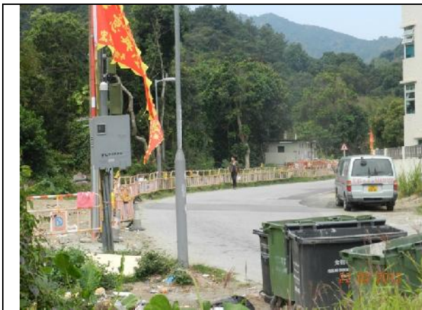
Photo 1 – Temporary hoardings have been erected around the active works area to the south of Wai Ha.
