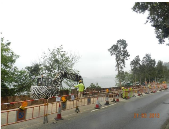
Photo 1 – Construction in a new section of road next to the main entrance of Area A was commenced.
