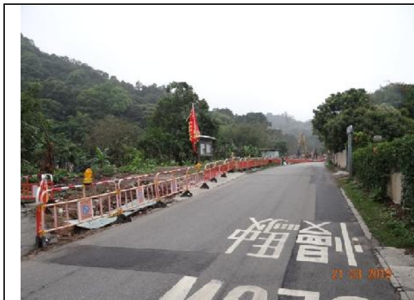
Photo 1 – Temporary hoardings have been erected along Tung Tsz Road near the refuse collection point opposite to Wai Ha.
