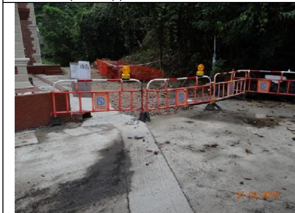
Photo 3 – Temporary hoardings have been erected on the path near Treasure Spot Garden II.
