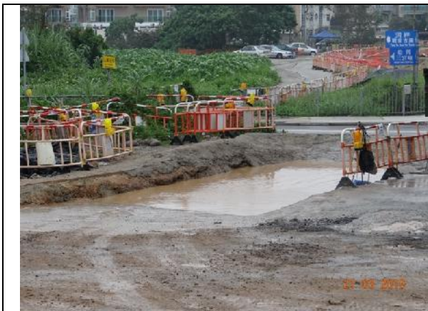
Photo 7 – Wheel washing facilities has been provided at the vehicular exit point of the works area of Contract 2.
