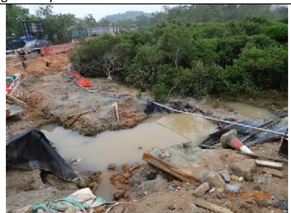
Photo 12 – The filtration tank opposite to San Tau Kok was removed and no more discharge was observed.
