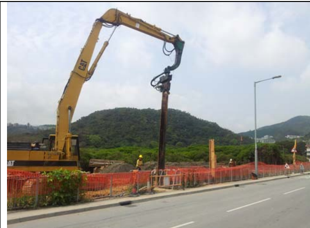
Photo 1: Rubber tube is missing at the chain of the vibration clip, the contractor was reminded to provide the rubber tube for the chain to reduce the noise level near the works area NSR.
