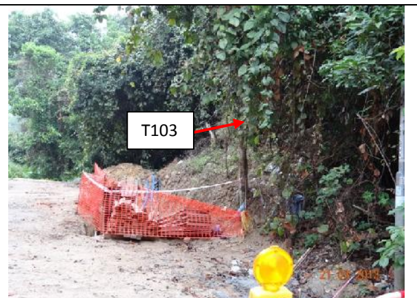
Photo 18 – The soil refilled to the retained tree T103 was loose and sandy, and tapes and ropes were found tied on the trunk.
