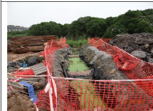
Photo 9 – The sedimentation beds with gravels and PVC liners was aligned from the area opposite to the Jade View Villa towards the marsh area at southeast.
