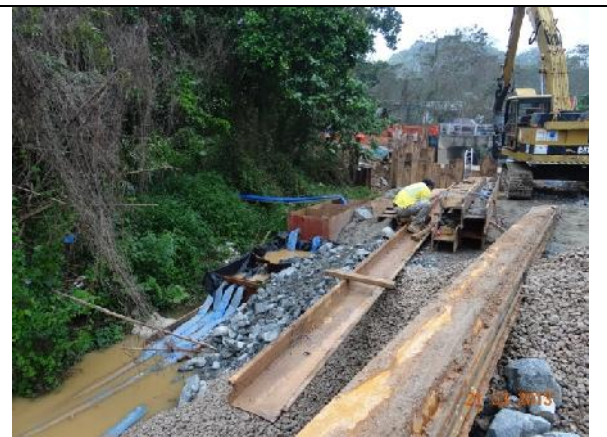
Photo 14 – The running water of the river was pumped to a sedimentation tank at the end of the works area.
