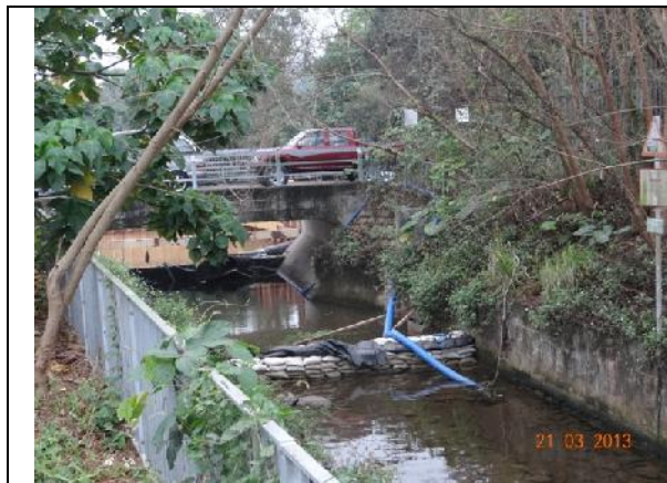
Photo 13 – Sand bags have been put in Wai Ha River to separate the works area in the river. The running water of the river was pumped to the end of the works area.
