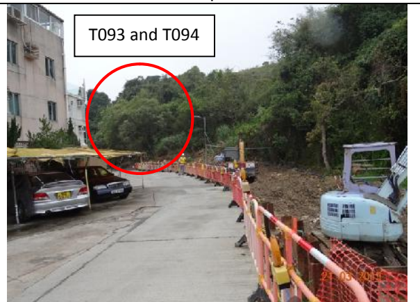
Photo 4 – Temporary hoardings have been extended to the northwest of the access road to Treasure Spot Garden II near retained trees T93 and T94.
