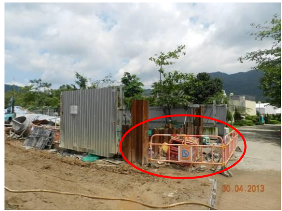
Photo 4 – The temporary hoardings at the eastern end of Phase 1 in the Nursery were replaced by temporary construction barriers.
