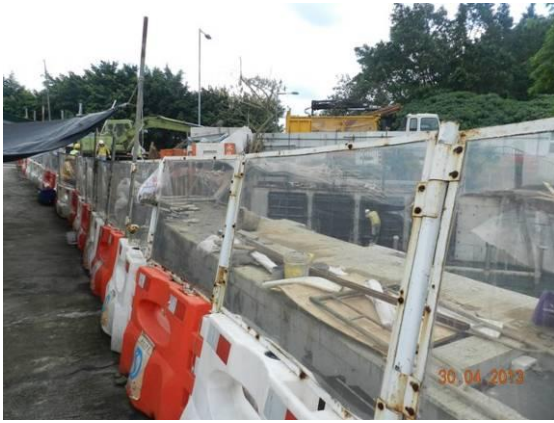
Photo 1 – Temporary hoardings have been established to surround the works area at Wai Ha River estuary.
