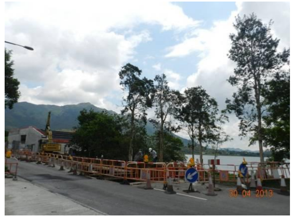
Photo 2 – Temporary barriers along a section of Ting Kok Road next to the main entrance of Area A.
