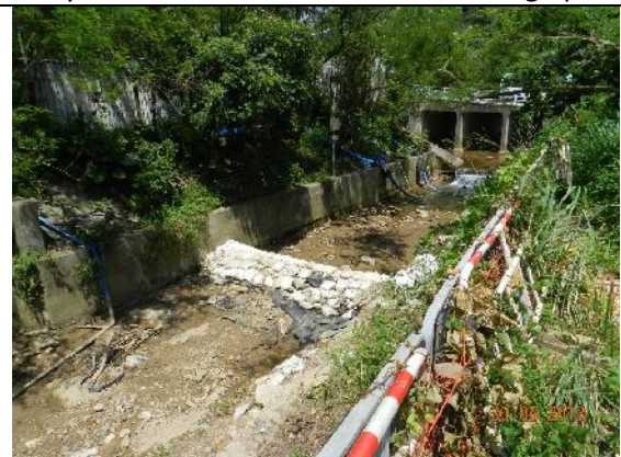
Photo 18 – Sand bags have been put in Wai Ha River to separate the works area in the river. The stream water was pumped to the end of the works area.
