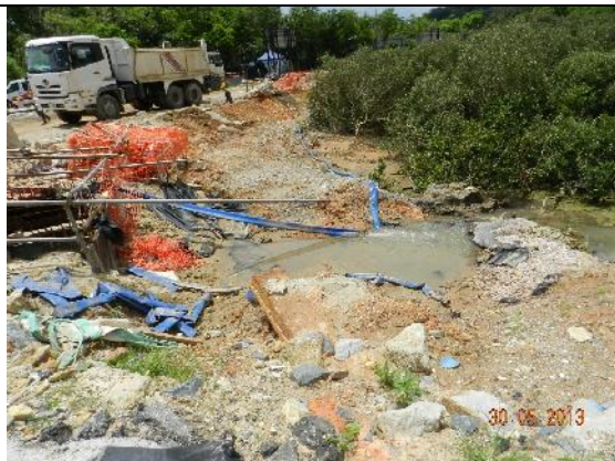
Photo 17 – Another section of sedimentation bed was aligned with PVC liner underlying granules close to the area at which a filtration tank was previously placed opposite to San Tau Kok close to the marsh area. The discharge is released to the marsh area but the discharge is not clean.
