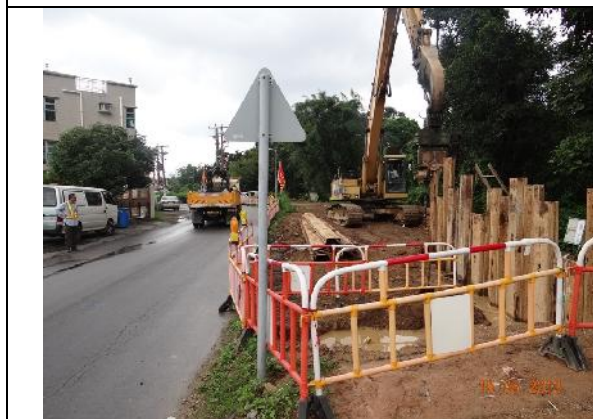
Photo 5 – Sheet piling was found in the construction site next to the public toilet on Tung Tsz Road on 15 th May 2013.
