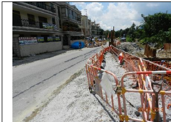
Photo 1 – Temporary hoardings have been erected along Tung Tsz Road opposite to Wai Ha.
