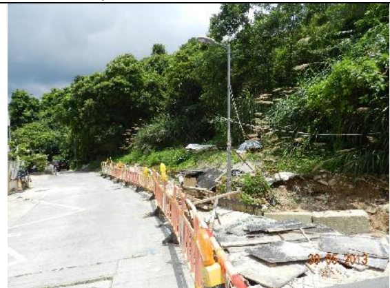
Photo 4 – Temporary hoardings have been extended to the northwest of the access road to Treasure Spot Garden II.
