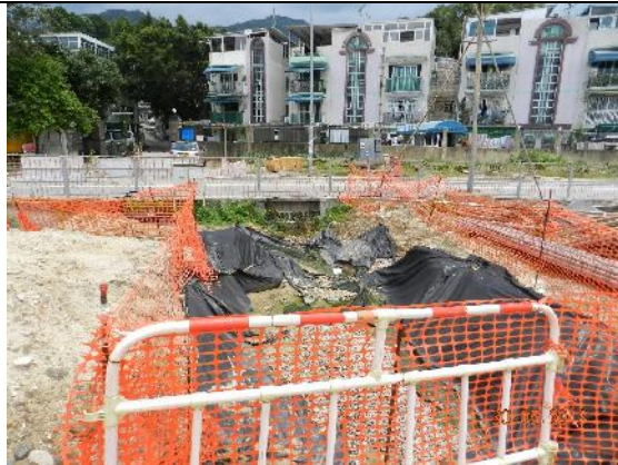
Photo 15 – The sedimentation beds with gravels and PVC liners were aligned from the area opposite to the eastern part of Jade View Villa towards the marsh area at southeast.
