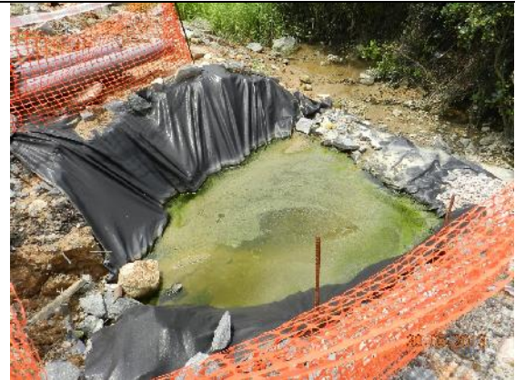
Photo 16 – A section of sedimentation bed has been aligned opposite to San Tau Kok with PVC liner underlying granules in April 2013. The discharge is released to the marsh area and no muddy water was observed at the drainage point.
