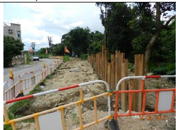
Photo 6 – No more work was found next to the public toilet on Tung Tsz Road on 30 th May 2013.
