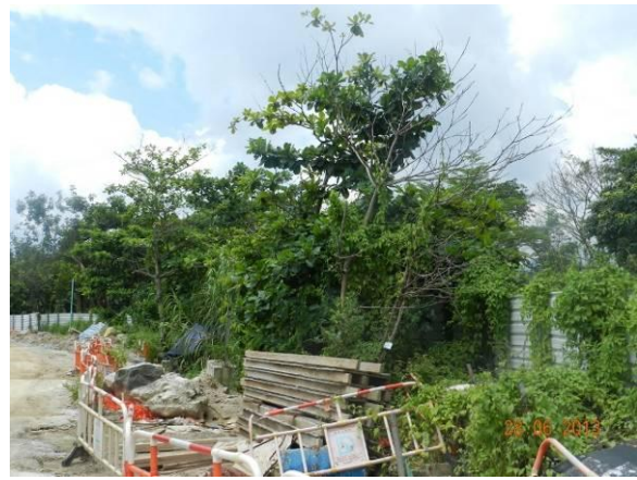
Photo 20 – Temporary storage of construction materials was observed close to the tree group of U34, U35, U37 and other trees in Area B.
