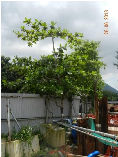
Photo 27 – Construction materials were found around the tree root zone of A42.
