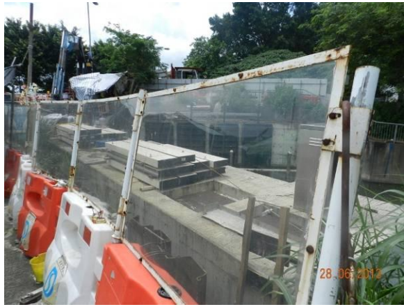
Photo 1 – Temporary hoardings have been established to surround the works area at Wai Ha River estuary.
