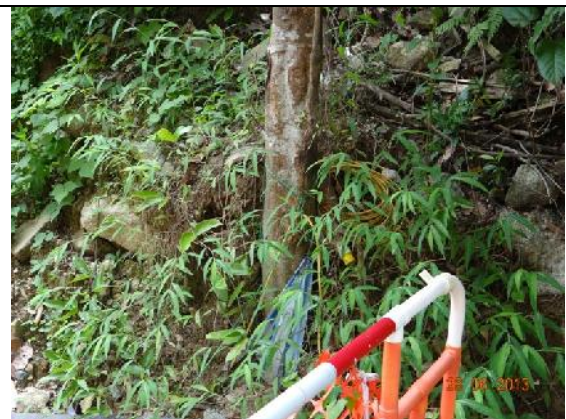
Photo 26 – The refilled soil at the trunk base of the retained tree T103 was loose and sandy, and tapes and ropes were still found tied on the trunk.
