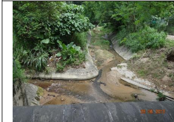
Photo 21 – No discharge of used water was observed at the upper section of Wai Ha River (i.e. to the north of Tung Tsz Shan Road).
