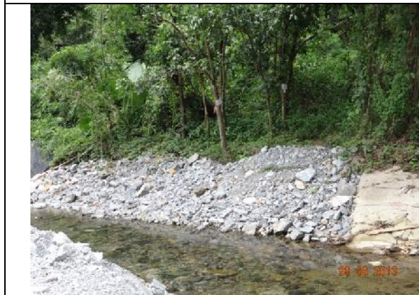
Photo 23 – The section of river bank with loose soil was refilled by stones and cobbles.
