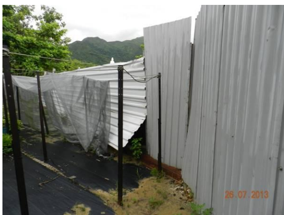
Photo 5 – No repair was observed on the broken section of site hoarding close to the retained tree U50 ( Ficus elastica ) at the southwestern part of Phase 1.
