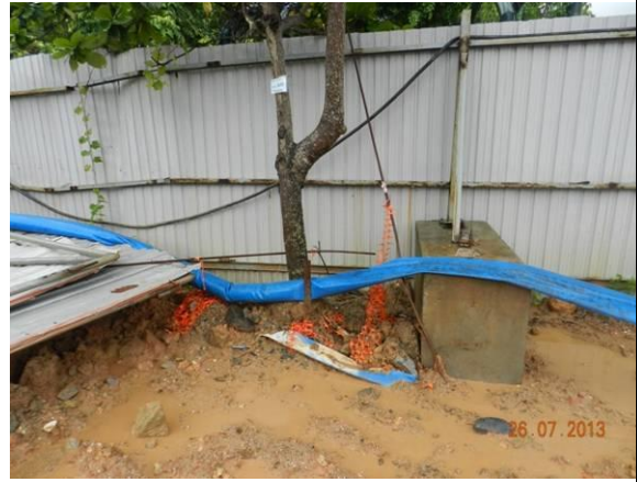
Photo 26 – Temporary stored construction materials were removed but soil piling was still observed close to the trunk flare of A43.
