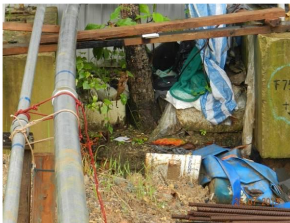
Photo 29 – Construction materials were found around the tree root zone of A42.
