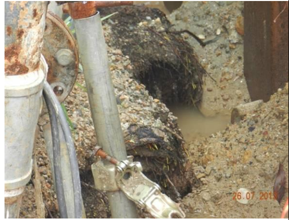
Photo 32 – Some of the tree roots growing underneath the tree planter of A40 could be damaged by the works.
