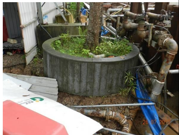
Photo 30 – Soil excavation works was observed around the planter of a retained tree A40 ( Terminalia catappa ) at the entrance of Phase 2 construction areas.
