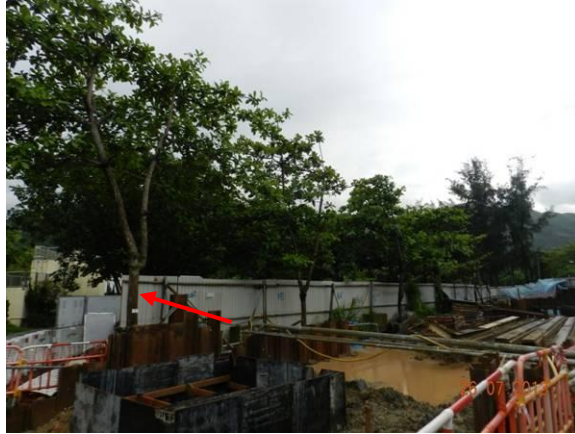
Photo 31 – The southern side of the tree planter of A40 has already been excavated for building the box culvert.
