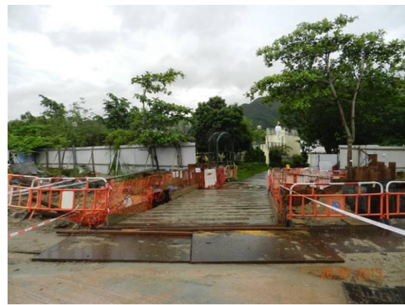
Photo 4 – The temporary hoardings at the eastern end of Phase 1 and the western end of Phase 2 works area were replaced by temporary construction barriers.
