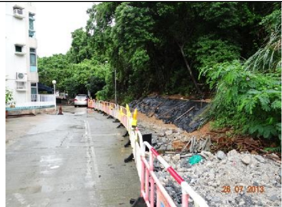
Photo 20 – Vegetation clearance was found near the tree group T93-T94.
