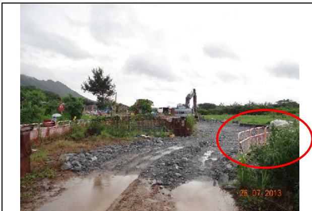
Photo 7 – Temporary construction barriers were erected to surround the eastern side of the wetland rehabilitation area,
