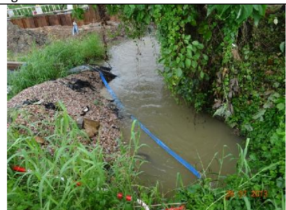
Photo 12 – Granules along the sedimentation beds and PVC liner near the retained tree T196 ( Macaranga tanarius var. tomentosa ) were removed and no muddy water was discharged.
