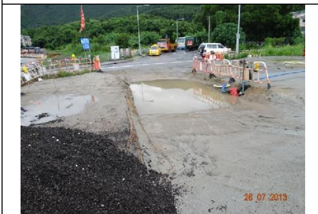
Photo 11 – Wheel washing facility has been provided at the vehicular exit point of the works area of Contract 2.
