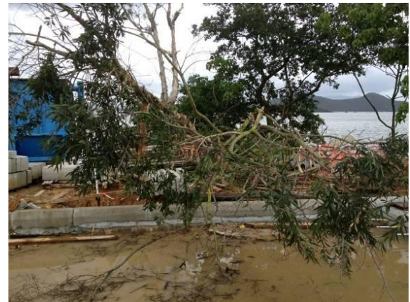
Photo 10 – Both relocated E18 and E97 collapsed under the strike of Typhoon Utor in August 2013. Photo is provided by the Main Contractor.
