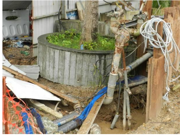
Photo 32 – The excavated area close to the retained tree A40 has not yet refilled as inspected in August 2013.
