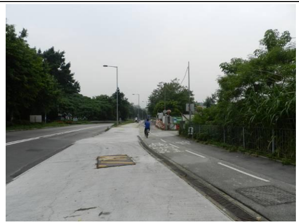
Photo 2 – The works area close to the estuary and located to the south of Area A along Ting Kok Road was completed in August 2013.
