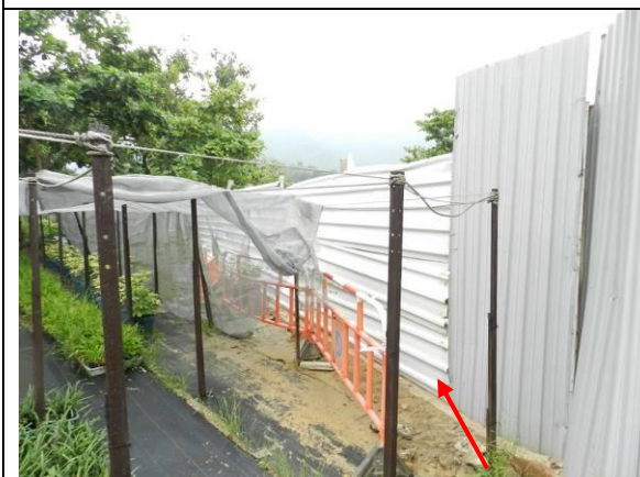
Photo 5 – A section of site hoarding close to the retained tree U50 at the southwestern part of Phase 1 was reinstated in August 2013.
