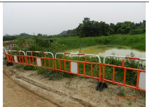
Photo 6 – Temporary construction barriers were seen surrounding the eastern side of the wetland rehabilitation area.
