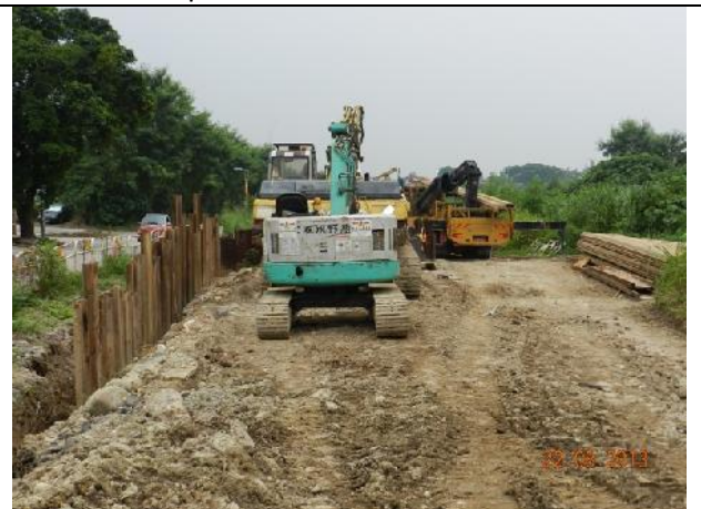
Photo 4 – Sheet piling work continued in the works area near the retained tree T190.
