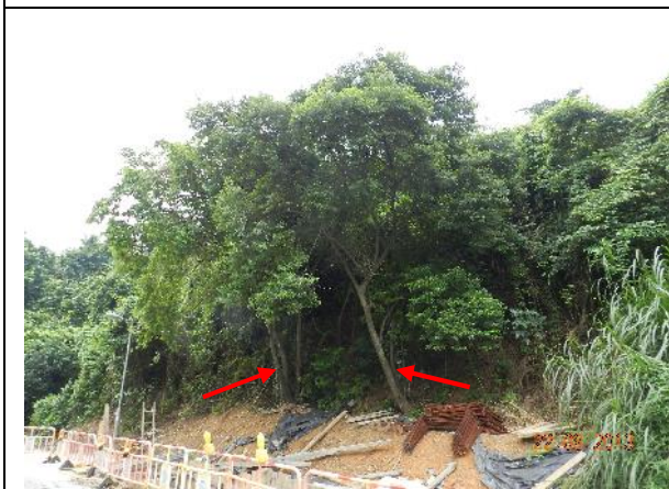
Photo 17 – Temporary storage of construction materials were noted close to the trunk flares and trunks of T093 and T094 (both indicated).
