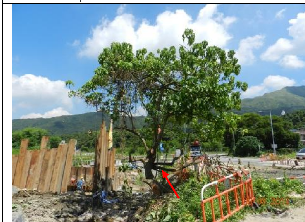
Photo 5 – Sheet piling work was seen close to the retained tree T196 (indicated).
