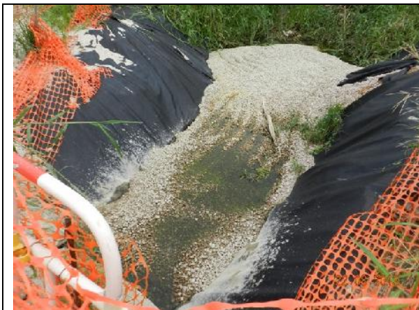
Photo 13 – A section of sedimentation beds aligned from the area opposite to the eastern part of Jade View Villa towards the marsh area. No muddy water was discharged.
