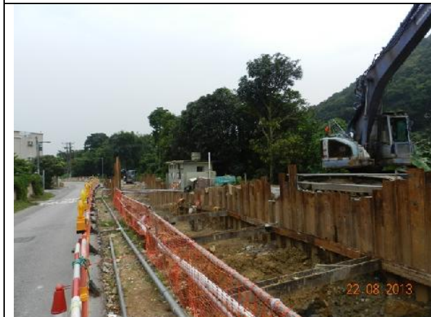
Photo 3 – Sheet piling work continued in the works area along Tung Tsz Road opposite to Wai Ha outside the public toilet.
