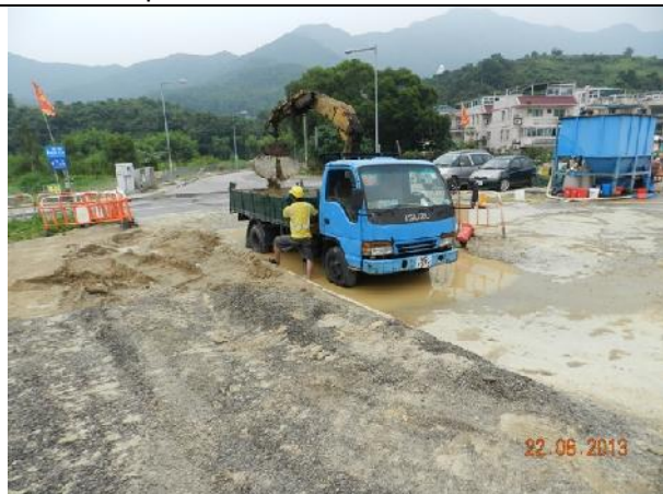
Photo 10 – Provision of wheel washing facilities noted at one major vehicular exit point of the works area of Contract 2.
