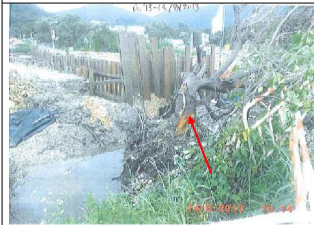
Photo 21 – The retained tree T196 was collapsed under the influence of Typhoon Utor hoisted on 14 th August 2013. This photo was provided by the Contractor.
