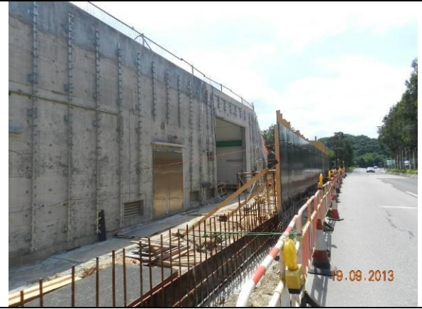
Photo 2 – The permanent boundary wall has started to be established along the western side of Area A.
