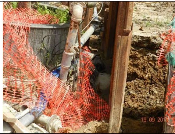
Photo 27 – The excavated area close to the retained tree A40 has not yet refilled as inspected in September 2013.
