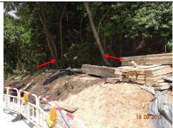
Photo 20 – Temporary storage of construction materials were still noted close to the trunk flares and trunks of T093 and T094 (both indicated).
