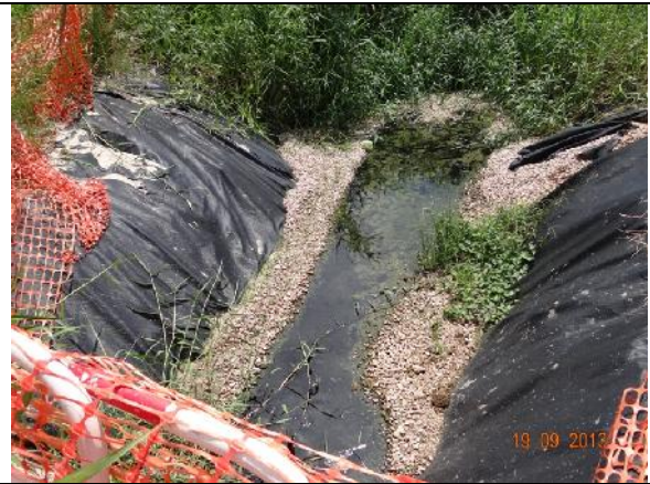
Photo 14 – A section of sedimentation beds aligned from the area opposite to the eastern part of Jade View Villa towards the marsh area. No muddy water was discharged.
