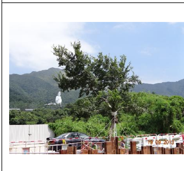
Photo 23 – The retained tree T025 was pruned before and it was temporarily guyed to provide additional support to this tree.
