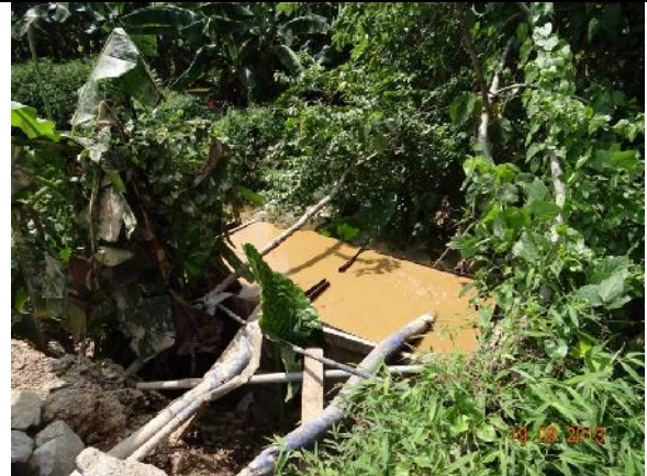
Photo 16 – A filtration tank was found on a slope near the public toilet on Tung Tsz Road. Muddy water from the works area was pumped to the filtration tank and the muddy water was seen overflowing and leaking into the stream.
