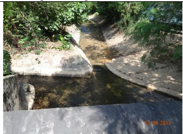
Photo 18 – No direct water discharge into the upper stream of Wai Ha River was observed as the construction works have been concentrated at the lower end of the river.
