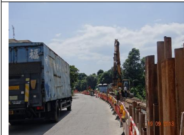
Photo 3 – Sheet piling work in the works area along Tung Tsz Road opposite to Wai Ha near the refuse collection point
