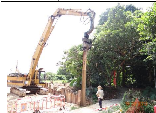
Photo 5 – Sheet piling work in the works area near the tree group T181-184.
