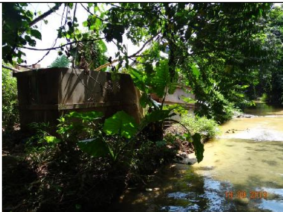
Photo 17 – Muddy water was seen overflowing and leaking into the stream.
