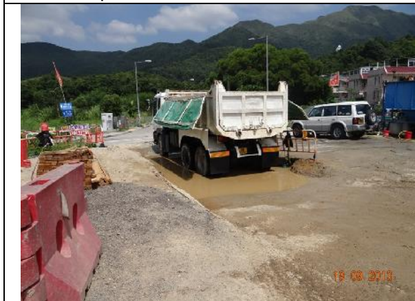
Photo 11 – Provision of wheel washing facilities was noted at one major vehicular exit point of the works area of Contract 2.
