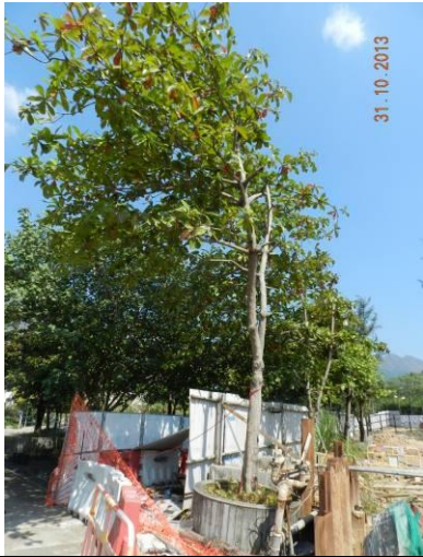
Photo 31 –The excavated area close to the planter of A40 has not yet refilled with soil.
