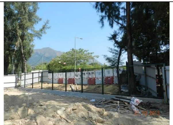
Photo 4 – Chain link fence was installed at the eastern end of Phase 2 works area.
