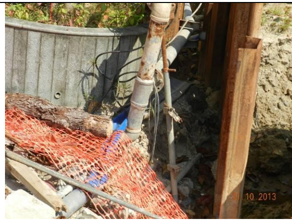
Photo 32 – The excavated area close to the planter of A40 has not yet refilled with soil.
