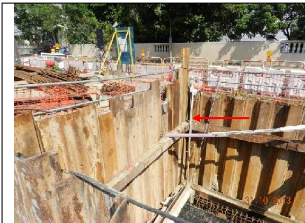
Photo 31 – Water from the box culvert in the works area outside the public toilet was noted pumping to a pipe next to Wai Ha River.
