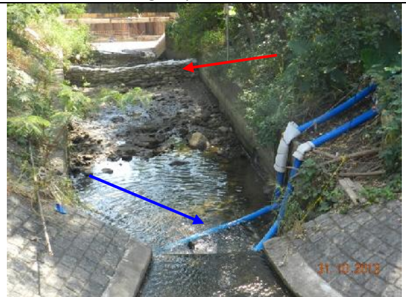
Photo 6 – The river was divided by sand bags (Red arrow) and water from the upper stream was pumped to the lower stream behind the works area along Wai Ha River (Blue arrow).
