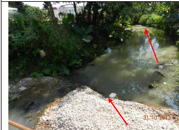
Photo 27 – Sections of granules with underlaid PVC liners were found along the river for further sedimentation.
