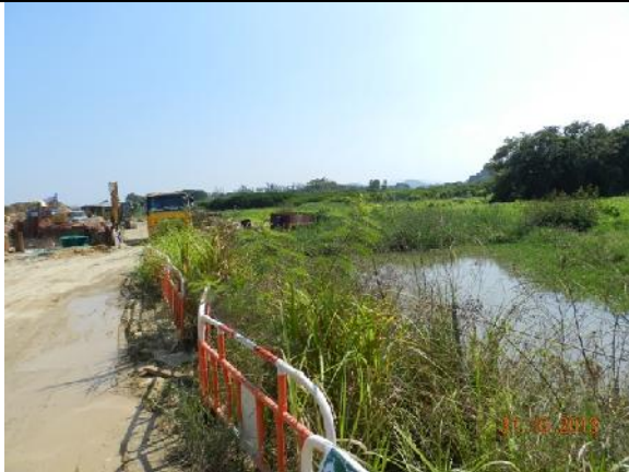
Photo 9 – Temporary construction barriers surrounding the eastern side of the wetland rehabilitation area.
