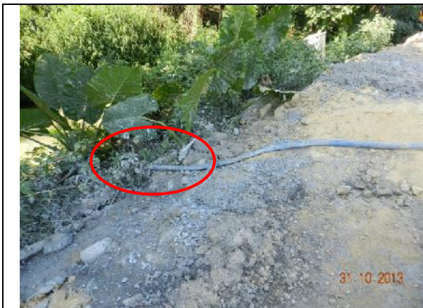
Photo 37 – Some muddy water from the box culvert in the works area was also found pumping to Wai Ha River directly.
