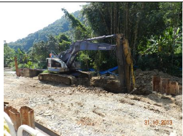
Photo 8 – Excavation works instead of sheet piling work in the works area along Wai Ha River on 31 st October 2013.
