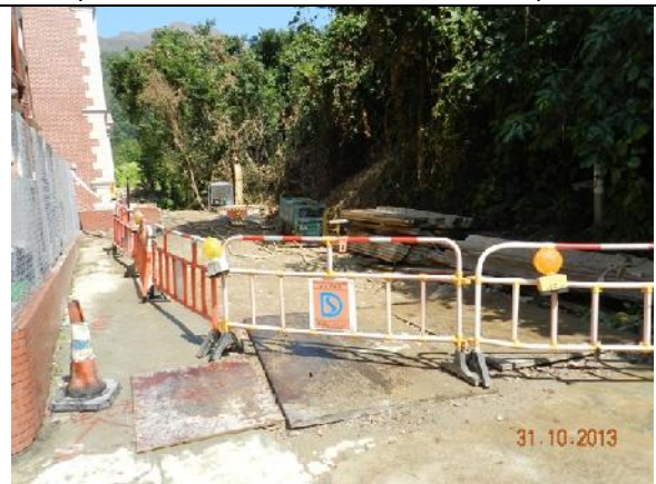
Photo 16 – Works were observed at the end of the Treasure Spot Garden II near the retained tree T103 and the works area was surrounded by temporary construction barriers.
