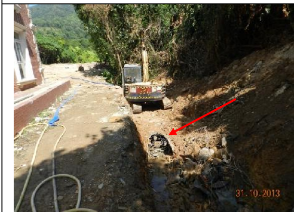
Photo 17 – Excavation work was noted at the end of the Treasure Spot Garden II for joining the old pipe (Red arrow) to the new box culvert.
