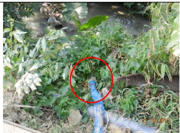
Photo 36 – Some muddy water from the box culvert in the works area was also found pumping to Wai Ha River directly.
