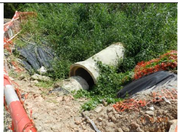
Photo 24 – A section of sedimentation bed aligned from the area opposite to the eastern part of Jade View Villa towards the marsh area. No muddy water was discharged.
