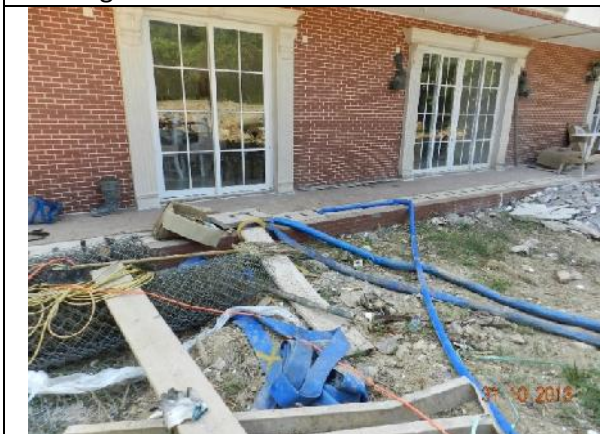
Photo 41 – Another view showing the pipes which pump the stream water from the stream to the drainage of the adjacent building.
