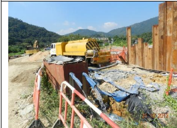
Photo 21 – A sedimentation tank receiving the waste water from the works area near the previous collapsed tree T196 ( Macaranga tanarius var. tomentosa ). Clear discharge was noted.
