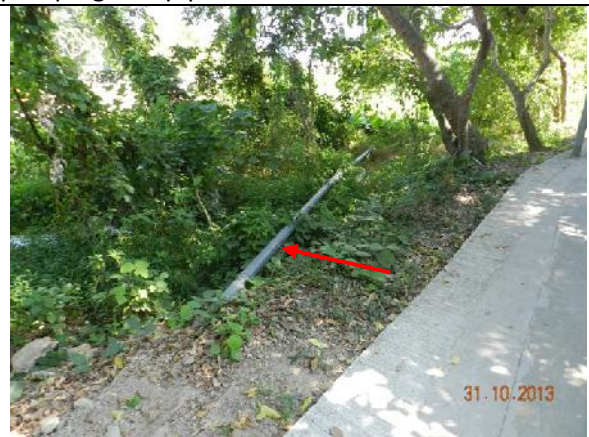
Photo 34 – The pipe was then directed along the river to the grassland behind the tree group T181-183.
