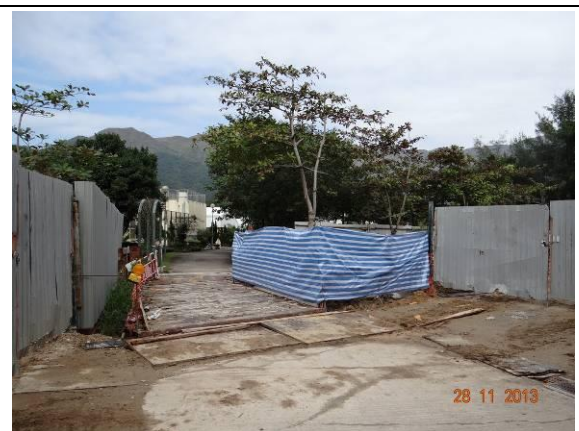
Photo 4 – The western end of Phase 2 of Area B was demarcated with temporary construction barriers and covered by canvas sheets.
