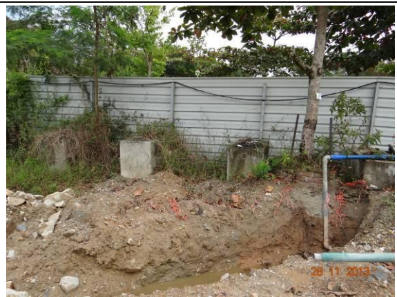
Photo 30 – Excavated holes have still existed next to the relocated trees.
