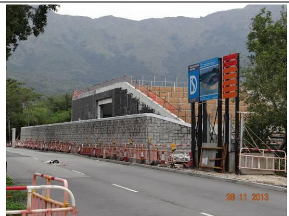
Photo 2 – The permanent boundary wall has been established along the western side of Area A.
