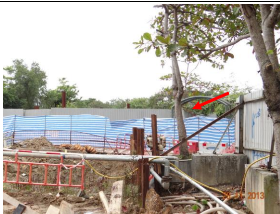
Photo 29 – Civil works close to the planter of A40 (indicated) were still on-going.
