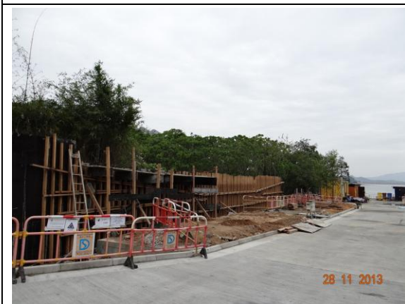
Photo 3 – The proposed boundary wall along part of the northern side of Area A was under construction.
