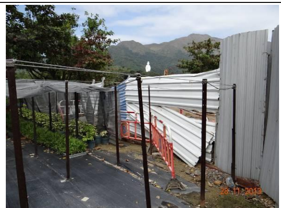
Photo 6 – A small section of the temporary hoarding at the southwestern side of Phase 1 works area of Area B was removed and covered by canvas sheets.
