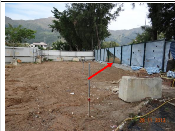
Photo 5 – Chain-link fence was reinstated at the eastern end of Phase 2 works area and covered by canvas sheets.
