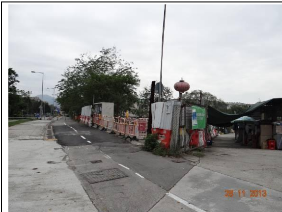
Photo 1 – Temporary hoardings have been established around the works area at Wai Ha River estuary.
