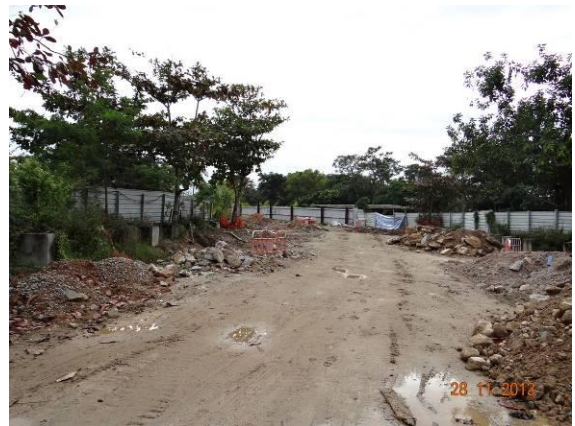
Photo 18 – Excavated soil was piled close to the relocated trees along both sides of Phase 1 area.
