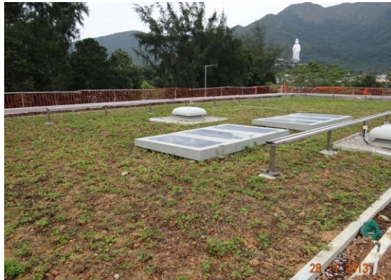
Photo 13 – Herbaceous creeper Arachis duranensis were planted on the green roof of the pump house.
