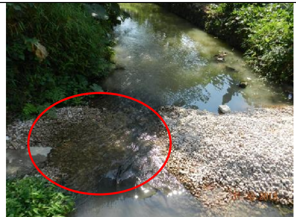
Photo 28 – Several sections of granules were washed away and the muddy water ran through it directly.
