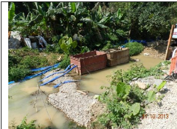
Photo 25 – The muddy water from the works area along Wai Ha River was pumped out from the river to a sedimentation tank settled at the end of the works area.
