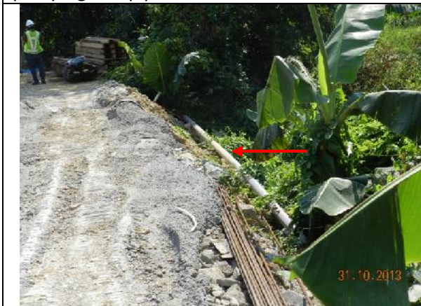
Photo 33 – The pipe was then directed along the river to the grassland behind the tree group T181-183.
