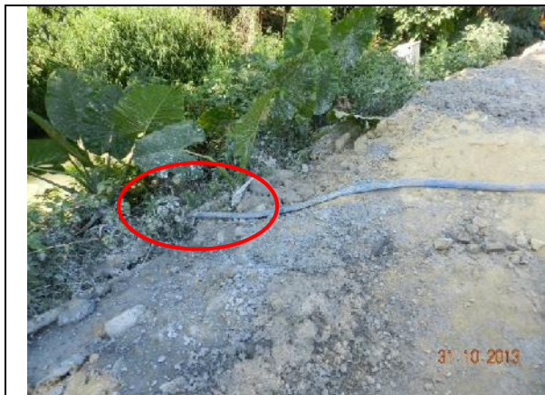
Photo 37 – Some muddy water from the box culvert in the works area was also found pumping to Wai Ha River directly.
