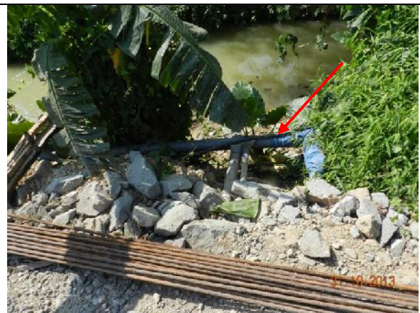
Photo 32 – Water from the box culvert in the works area outside the public toilet was noted pumping to a pipe next to Wai Ha River.
