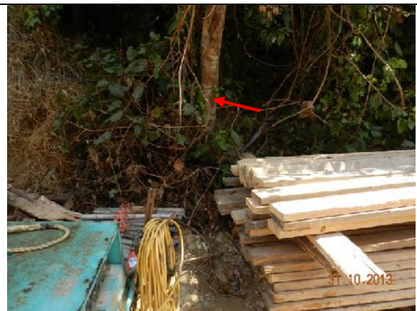
Photo 50 – Stockpiling were noted close to the trunk base of the retained tree T103.
