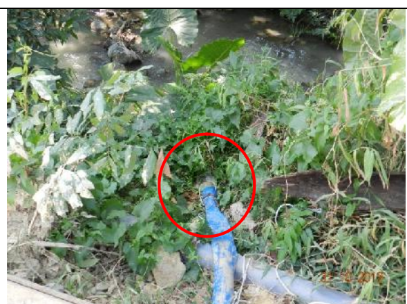
Photo 36 – Some muddy water from the box culvert in the works area was also found pumping to Wai Ha River directly.
