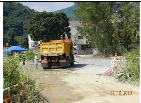
Photo 20 – A new exit for Contract 2 works area was seen opposite to the tree group T021-029 ( Leucaena leucocephala ) and workers were noted washing the wheels of the vehicles which were leaving the works area.
