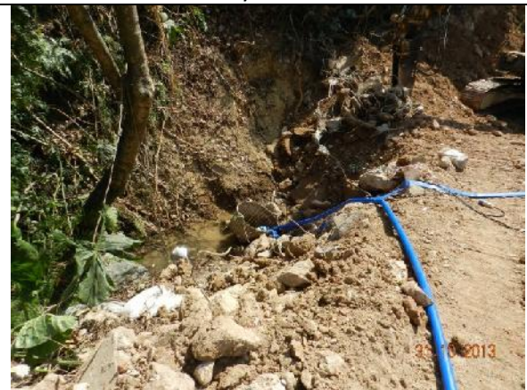
Photo 40 – The stream water was pumped to the drainage of the adjacent building.
