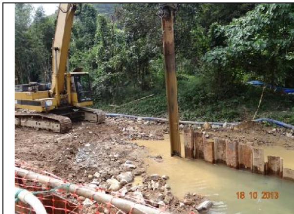
Photo 7 – Sheet piling work in the works area along Wai Ha River on 18 th October 2013.
