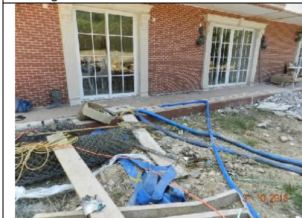
Photo 41 – Another view showing the pipes which pump the stream water from the stream to the drainage of the adjacent building.
