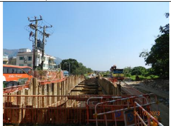
Photo 4 – Construction works for building the box culverts along Tung Tsz Road opposite to Wai Ha and near the tree group T181-184.
