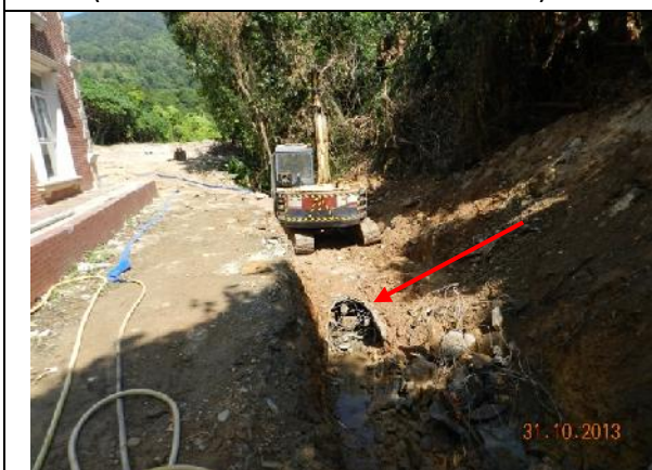
Photo 17 – Excavation work was noted at the end of the Treasure Spot Garden II for joining the old pipe (Red arrow) to the new box culvert.
