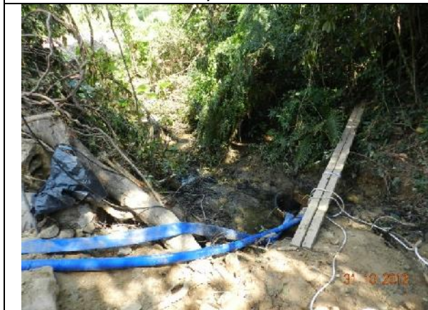
Photo 39 – In the works area at the end of the Treasure Spot Garden II next to the retained tree T103, a stream was blocked and the stream water was pumped to the drainage of the adjacent building.
