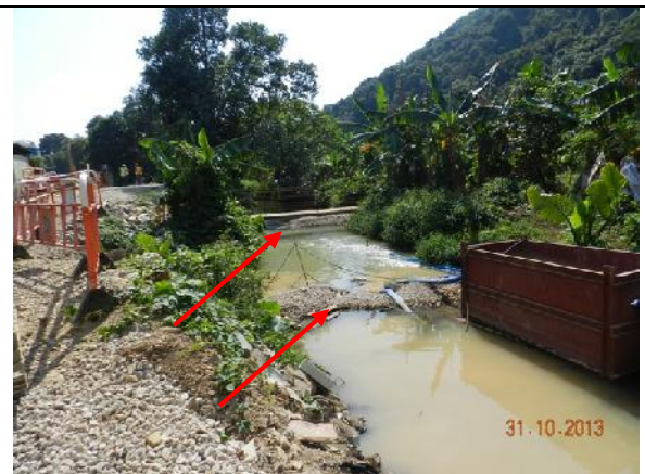
Photo 26 – Sections of granules with underlaid PVC liners were found along the river for further sedimentation.
