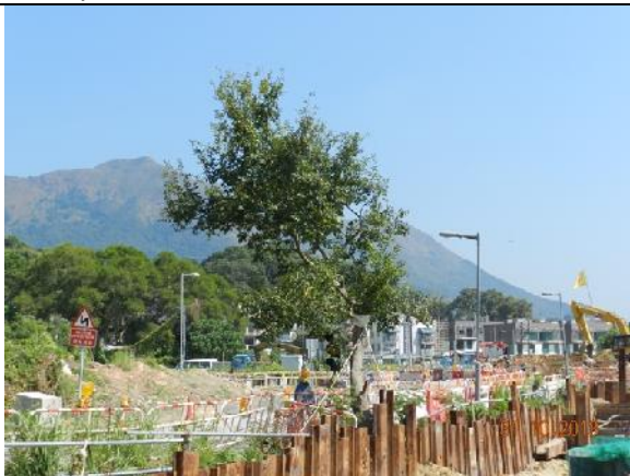
Photo 51 – The retained tree T025 was pruned before and it was temporarily guyed to provide additional support to this tree.
