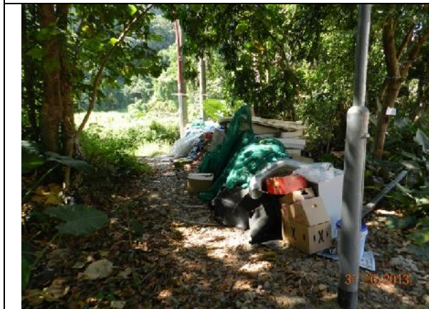
Photo 11 – Temporary storage of construction materials next to the retained tree T179 in October 2013.
