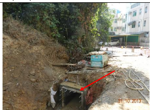
Photo 18 – Excavation work was noted at the end of the Treasure Spot Garden II for joining the old pipe to the new box culvert (Red arrow).
