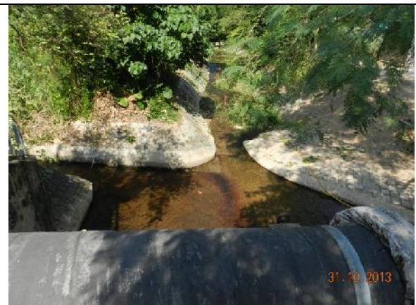
Photo 42 – No direct water discharge into the upper stream of Wai Ha River was observed as the construction works have been concentrated at the lower end of the river.
