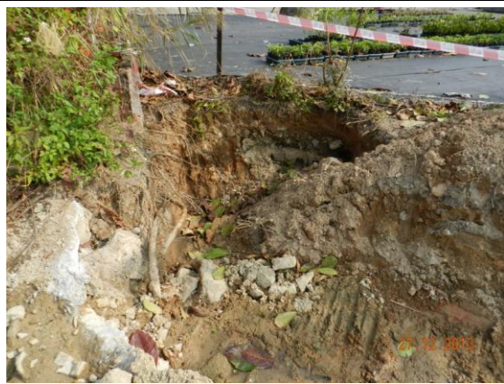
Photo 9 – Minor excavation works were undertaken in Phase 1 to reinstate the irrigation pipes.
