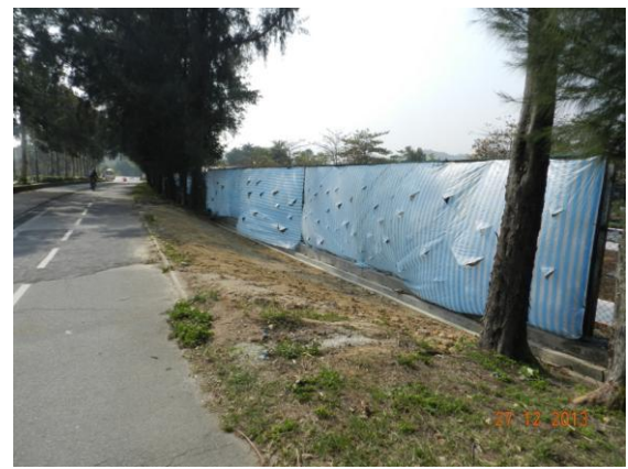
Photo 6 – Chain-link fence was reinstated at the eastern end of Phase 2 works area and covered by canvas sheets.
