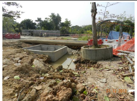
Photo 28 – The excavated area close to the planter of A40 has not yet refilled with soil.
