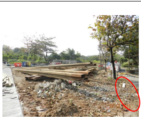
Photo 26 – U76, U78 and U79 were removed and their original locations were indicated in photo.
