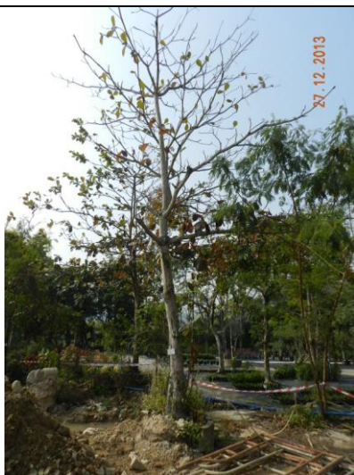
Photo 23 – Half of the planter of U47 was broken, but was not yet repaired.
