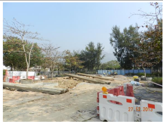
Photo 10 – The reinstatement works for the original access paths and ground of the nursery beds were in progress
