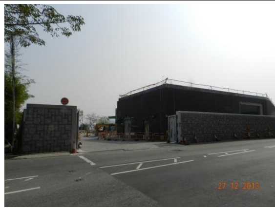
Photo 3 – Construction of the proposed boundary walls along part of the northern and western sides of Area A was in progress.
