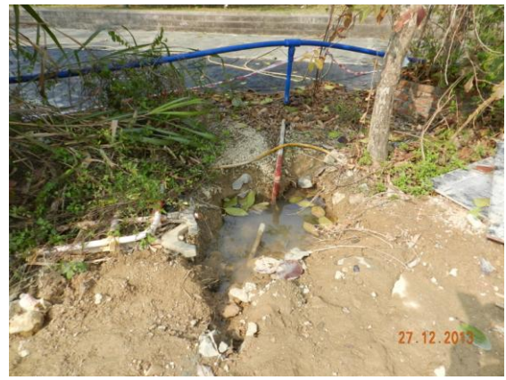
Photo 8 – Minor excavation works were undertaken in Phase 1 to reinstate the irrigation pipes.
