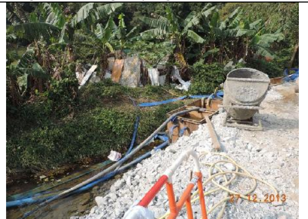
Photo 16 – The muddy water from the works area was pumped out from the river and back to a sedimentation tank settled at the end of the works area.
