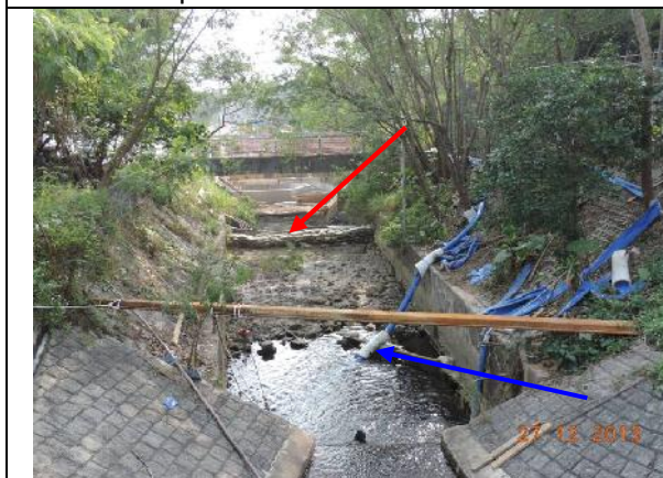
Photo 5 – The river was divided by sand bags (Red arrow) and water from the upper stream was pumped to the lower stream behind the works area along Wai Ha River (Blue arrow).
