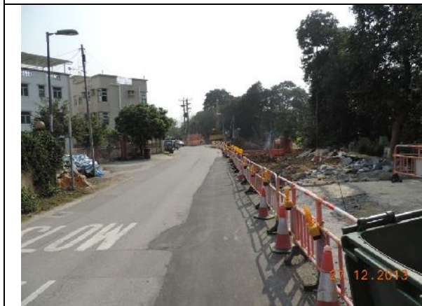
Photo 3 – Construction work for building the box culverts along Tung Tsz Road opposite to Wai Ha outside the public toilet.
