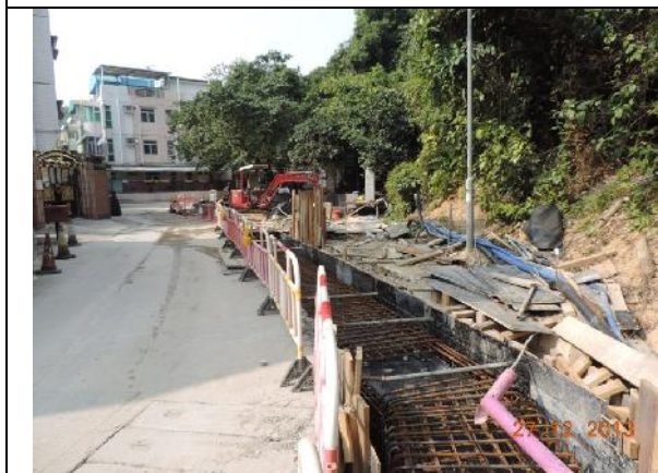
Photo 11 – Active construction works were also seen on the pathway to the Treasure Spot Garden II near the retained tree group (T097-098).
