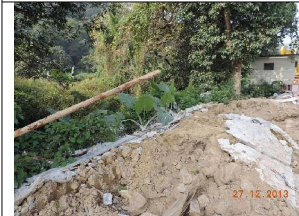
Photo 21 – In the works area near the public toilet, cement mortar and surplus soil were spread onto the slope and the vegetation next to Wai Ha River.
