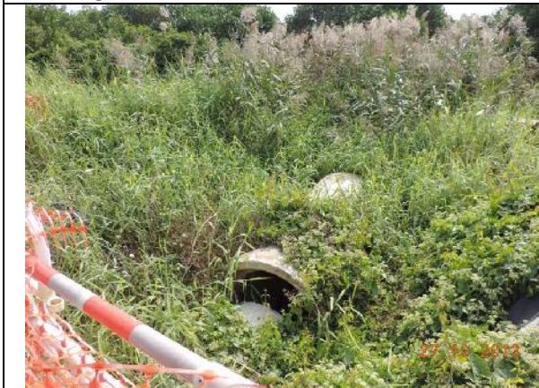
Photo 15 – Abandoned sedimentation bed aligned from the area opposite to the eastern part of Jade View Villa towards the marsh area with overgrown dense grassy vegetation.
