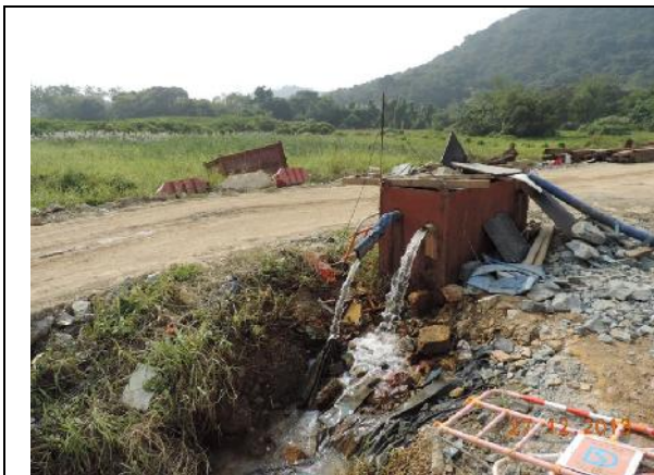
Photo 13 – A sedimentation tank was seen receiving the waste water from the works area near the previous collapsed tree T196 and the discharge was seen to be clear.
