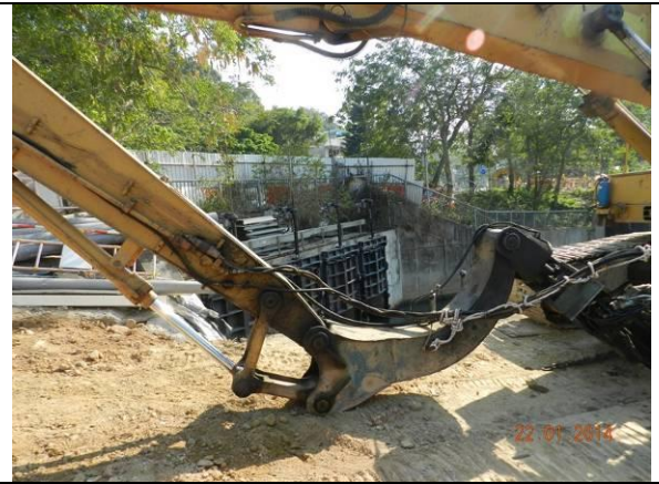
Photo 2 – Temporary construction hoardings have been established around the works area at Wai Ha River estuary.
