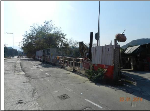
Photo 1 – Temporary construction hoardings have been established around the works area at Wai Ha River estuary.
