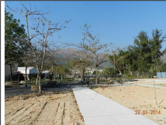
Photo 7 – The open section between Phases 1 and 2 work areas was opened again after the reinstatement works.
