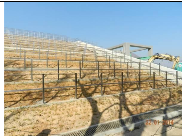
Photo 12 – The proposed green roof of the pumping house was vegetated with ground cover Arachis duranensis .
