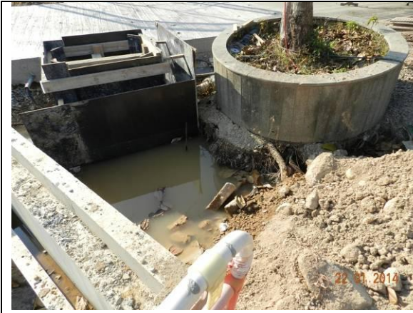
Photo 31 – The excavated area close to the planter of A40 has not yet been refilled with soil.
