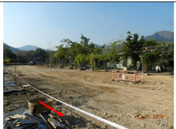
Photo 6 – The temporary construction hoardings in Phase 1 were removed and replaced by barrier tape.
