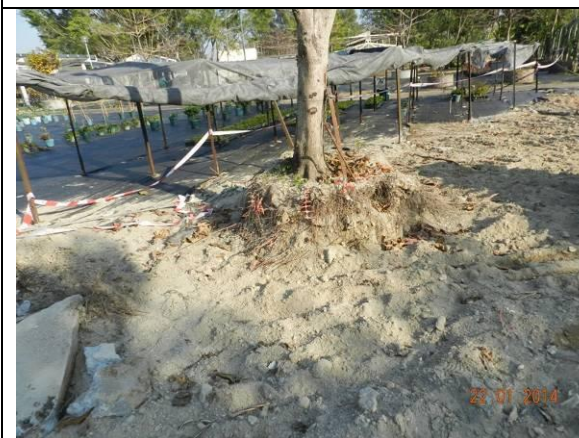
Photo 27 – The planter of another untagged Terminalia catappa next to U54 was broken, with exposed roots and soil.
