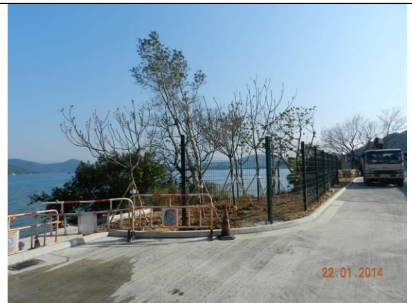
Photo 4 – Proposed chain-link fence has partly erected along the rest of the boundary sides of Area A.
