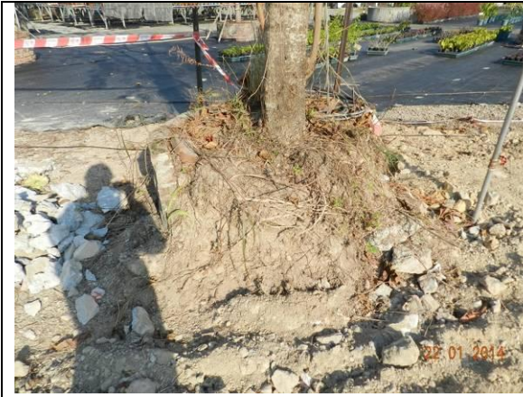
Photo 25 – The planter of U54 was broken and exposed roots and soil were observed.
