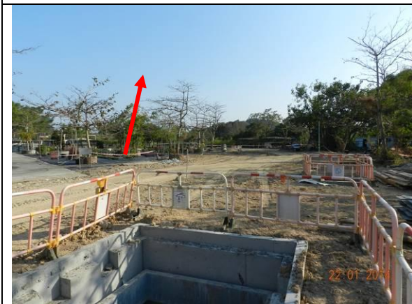
Photo 5 – The temporary construction hoardings in Phase 1 were removed and replaced by barrier tape.
