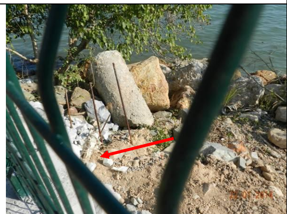
Photo 18 – The leaning E61 was removed in January 2014. Its original location is indicated.
