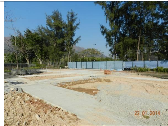
Photo 10 – The reinstatement works for the original access paths and ground of the nursery beds were about to be finished in Phase 2.
