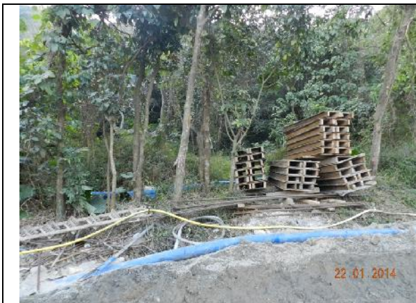
Photo 31 – No more stockpiling of construction materials was found touching the trunk flares of the tree group (T119-122) next to the works area in Wai Ha River, however these materials were relocated and put within the tree dripline area.
