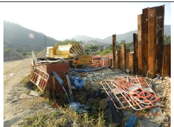
Photo 14 – A sedimentation tank was seen receiving the waste water from the works area near the previous collapsed tree T196 and the discharge was seen to be clear.
