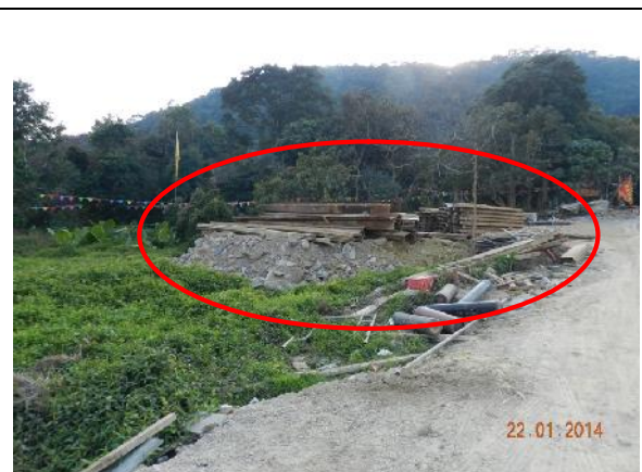
Photo 12 – The works area near the previous collapsed tree T190 ( Ficus hispida ) was found to be expanded to the grassland on the southern side. The expanded area was seen to be used for storage of construction materials.
