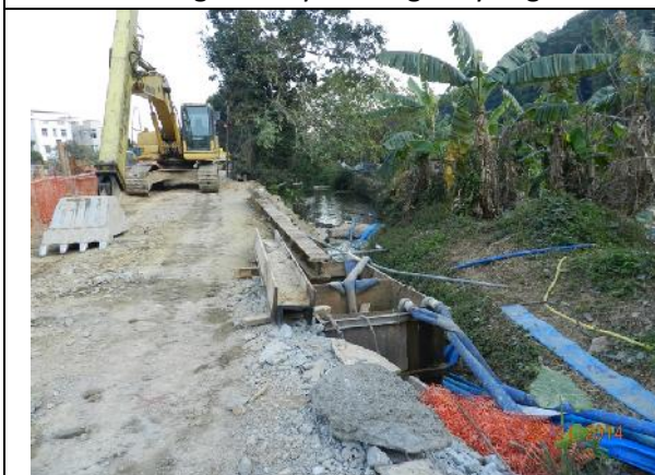
Photo 17 – The muddy water from the works area was pumped out from the river and back to a sedimentation tank settled at the end of the works area.
