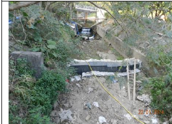
Photo 5 – The river was divided by sand bags and water from the upper stream was pumped to the lower stream behind the works area along Wai Ha River.
