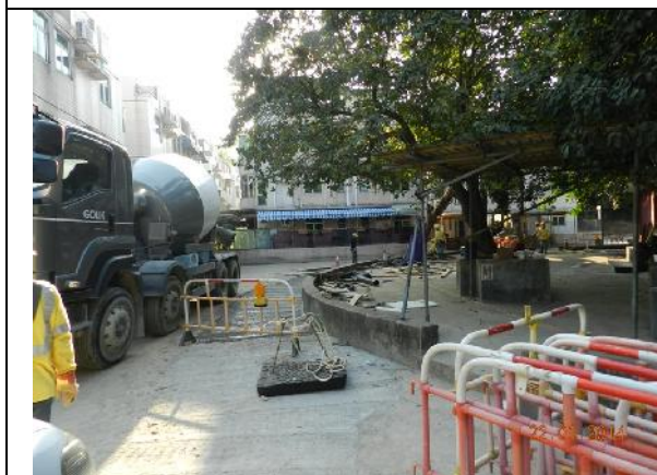
Photo 11 – Construction works were almost finished on the pathway to the Treasure Spot Garden II near the retained tree group (T097-098).
