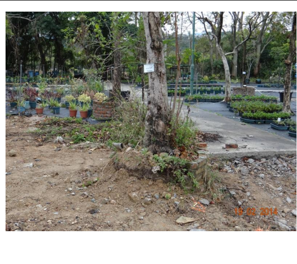
Photo 24 – Half of the planter of U47 was broken, but has not yet been repaired.
