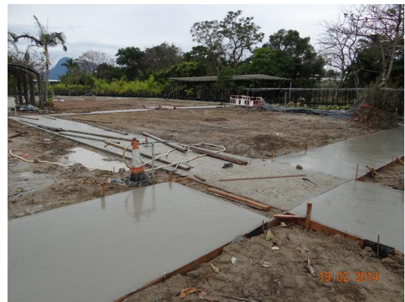
Photo 12 – The reinstatement works for the original access paths and ground of the nursery beds in Phase 1 area in Area B.
