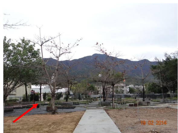
Photo 6 – The temporary construction hoardings in Phase 1 were removed and replaced by barrier tape (red arrow).
