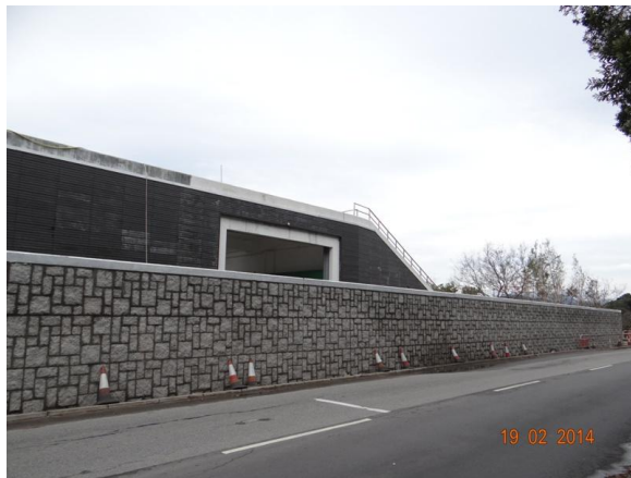
Photo 3 – Construction of the proposed boundary walls along part of the northern and western sides of Area A was finished.
