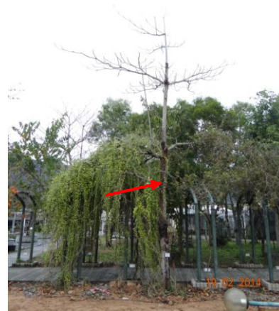
Photo 34 – The trunk of the transplanted tree U53 was tied tightly by strings and a hessian wrapping which was left after the transplantation of the tree.
