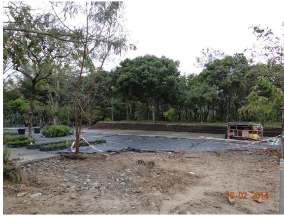
Photo 7 – The temporary construction hoardings in Phase 1 were removed and replaced by barrier tape. Some tapes were not firmly tied.
