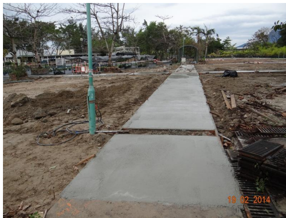
Photo 11 – The reinstatement works for the original access paths and ground of the nursery beds in Phase 1 area in Area B.
