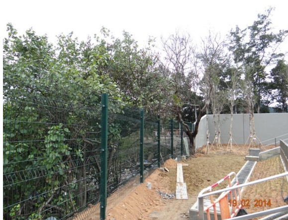
Photo 5 – Proposed chain-link fence has been erected along the rest of the boundary sides of Area A.
