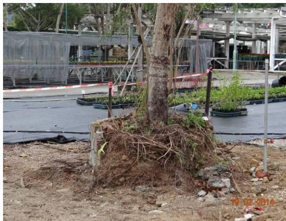
Photo 27 – The planter of U54 was broken and exposed roots and soil were observed.
