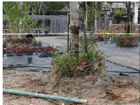
Photo 28 – The planter of an untagged Terminalia catappa next to U54 was broken, with exposed roots and soil.
