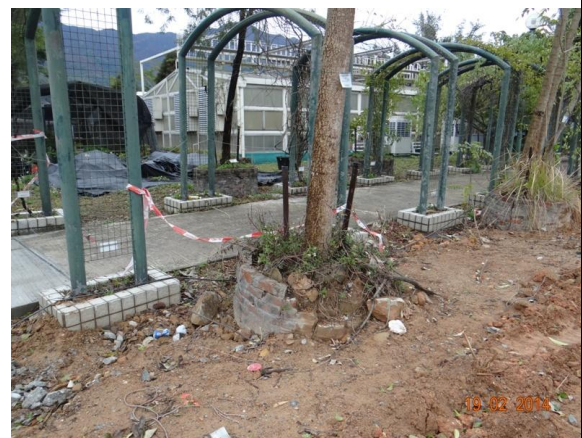
Photo 30 – The planter of U69 was broken and exposed roots and soil were observed.
