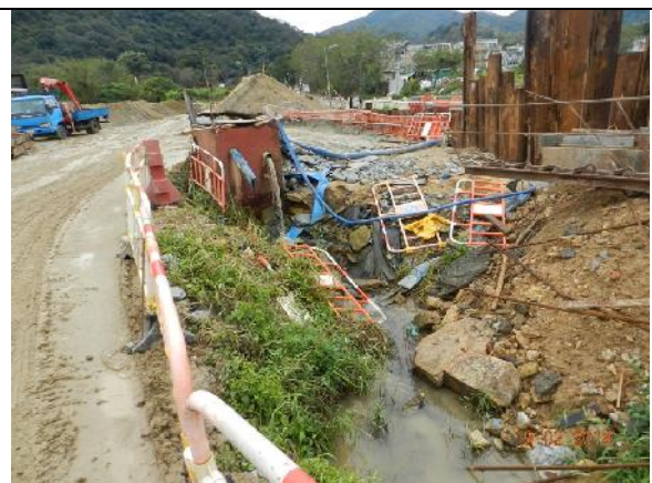
Photo 12 – A sedimentation tank was seen receiving the waste water from the works area near the previous collapsed tree T196 and the discharge was seen to be clear.
