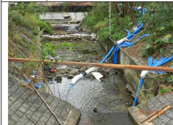
Photo 5 – The river was divided by sand bags and water from the upper stream was pumped to the lower stream behind the works area along Wai Ha River.
