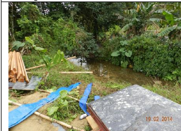
Photo 21 – No more water from the box culvert in the works area outside the public toilet was noted pumping out and releasing to Wai Ha River.
