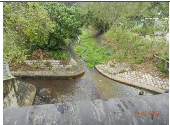
Photo 22 – No direct water discharge into the upper stream of Wai Ha River was observed as the construction works have been concentrated at the lower end of the river.
