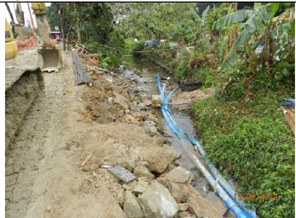
Photo 16 – The river water from the upper stream was released back to the river near the sedimentation tank.
