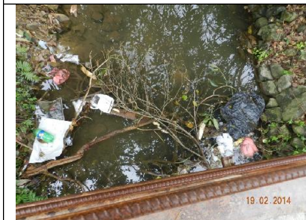
Photo 17 – Down the stream near the public toilet, broken branches from the adjacent trees were noted blocking the stream.
