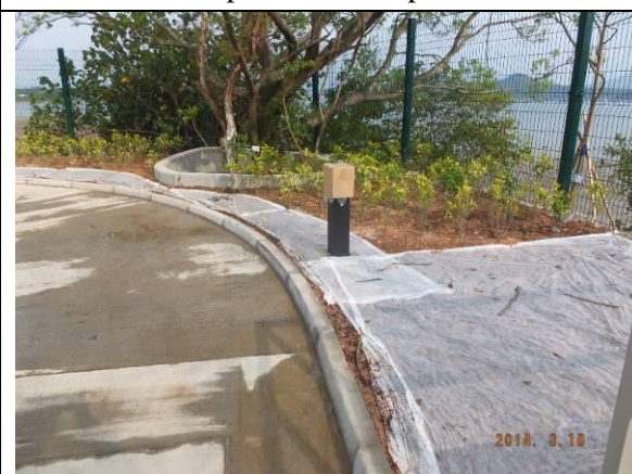
Photo 18 – Planting of shrubs and hydroseeding were observed in the newly built planters in Area A.
