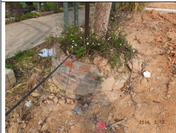
Photo 27 – The planter of U69 was broken and exposed roots and soil were observed. A risk of leaning tree trunk was observed.
