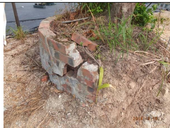
Photo 24 – The planter of U54 was broken and exposed roots and soil were observed.
