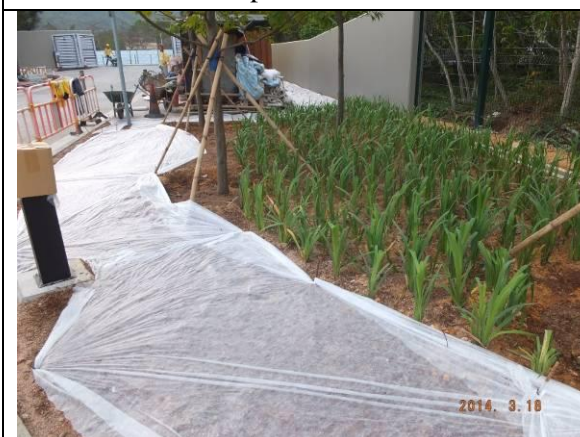
Photo 17 – Planting of shrubs and hydroseeding were observed in the newly built planters in Area A.
