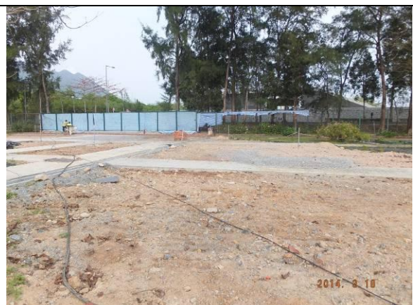
Photo 6 – The reinstatement works continued in Phase 2 of Area B within Tung Tze Nursery.
