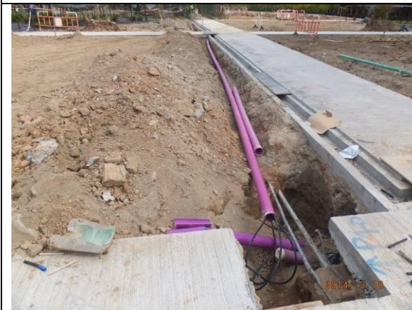
Photo 9 – The reinstatement works for the ground of the nursery beds and basic nursery utility were still in progress in both Phases 1 and 2 areas in Area B.
