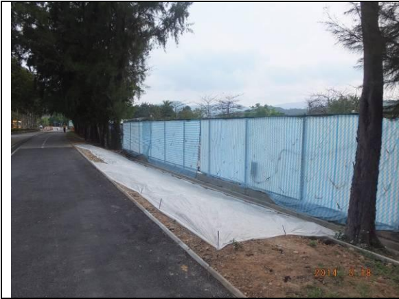
Photo 7 – Chain-link fence was reinstated at the eastern end of Phase 2 works area and covered by canvas sheets. Hydroseeding was applied on a roadside planting area next to Ting Kok Road.
