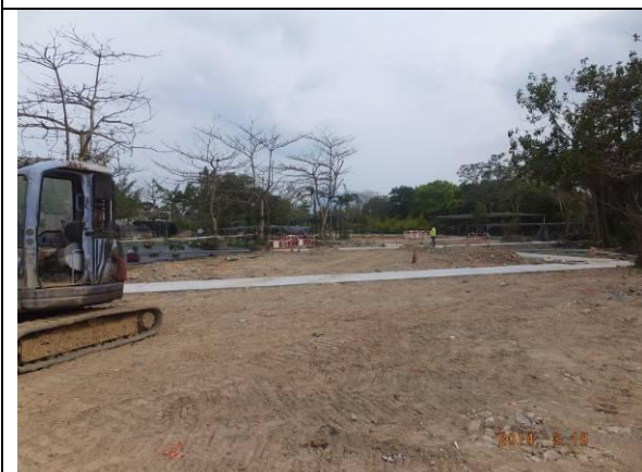
Photo 5 – The reinstatement works continued in Area B and the areas were demarcated with loosened barrier tapes.
