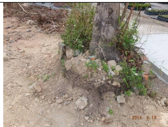
Photo 23 – Half of the planter of U47 was broken, but has not yet been repaired.
