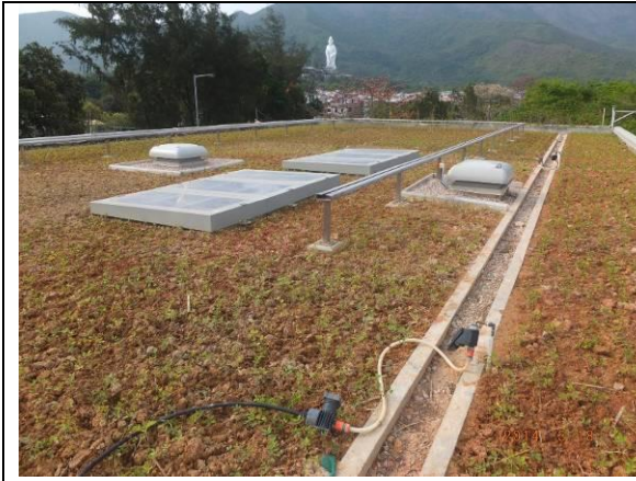
Photo 13 – The rooftop of the pumping house was vegetated with ground cover Arachis duranensis .
