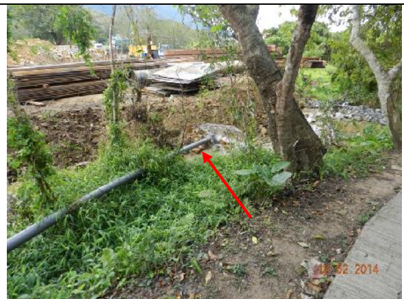
Photo 20 – Another view showing the water pumped from the nearby box culvert and released to the southern side of the area.
