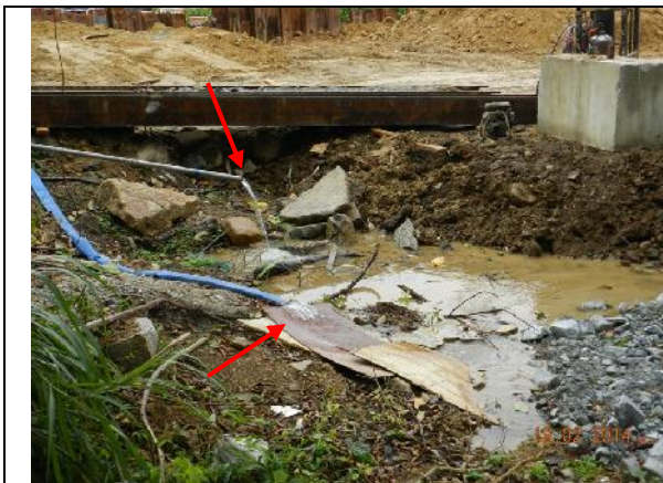
Photo 19 – Next to the expanded works area near the previous collapsed tree T190, water from the nearby box culvert was found pumping out and releasing to the southern side of the area.
