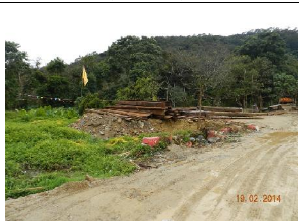
Photo 10 – The expanded works area near the previous collapsed tree T190 ( Ficus hispida ) was still used for storage of construction materials.
