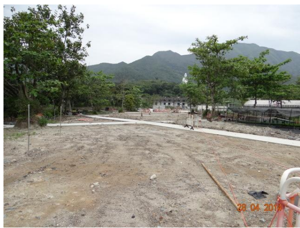
Photo 6 – Phase 1 area of Area B was demarcated by loosened barrier tape.
