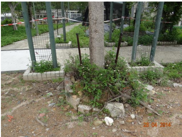
Photo 27 – The planter of U69 was broken and the exposed roots and soil were observed.
