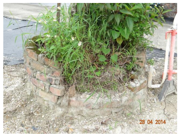
Photo 24 – The planter of U54 was broken and the exposed roots and soil were observed.
