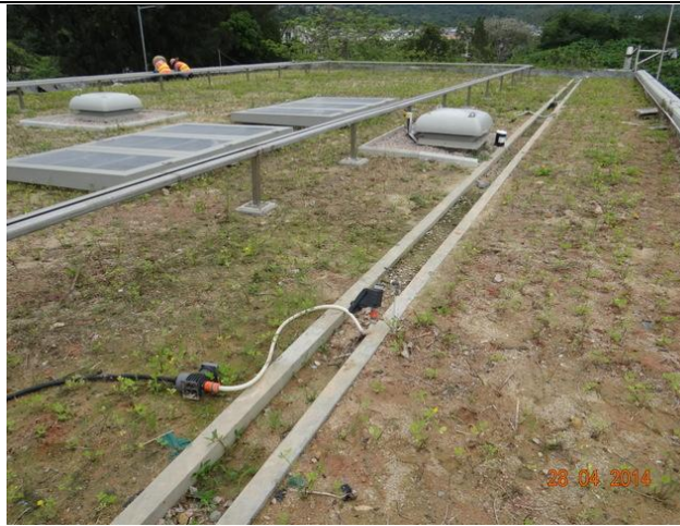
Photo 13 – No significant damage was observed on the rooftop of the pumping house.
