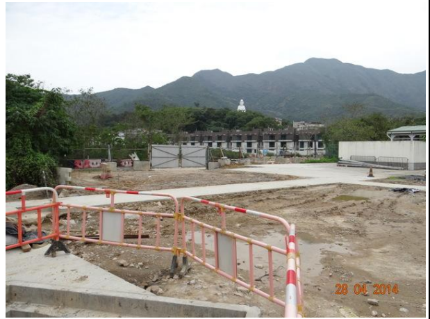
Photo 10 – The reinstatement works for the ground of the nursery beds and basic nursery utility were still under progress in both Phases 1 and 2 areas in Area B.
