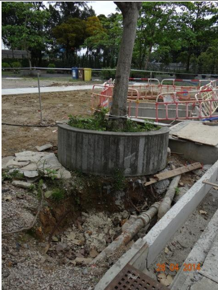
Photo 31 – The northern excavated area close to the planter of the retained tree A40 was not yet refilled.
