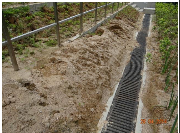
Photo 12 – Some soil which was washed away from the slanting component of the pumping house was removed subsequently.
