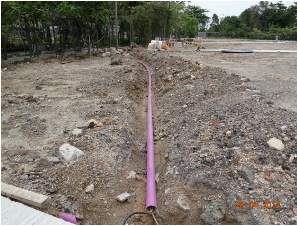
Photo 9 – The reinstatement work for the basic nursery utility was still under progress in Phase 1 area of Area B.
