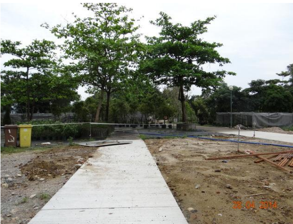
Photo 5 – The reinstatement work in Phase 2 area of Area B was demarcated by barrier tape.
