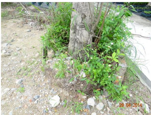
Photo 23 – Close-up view of the broken planter of U47.
