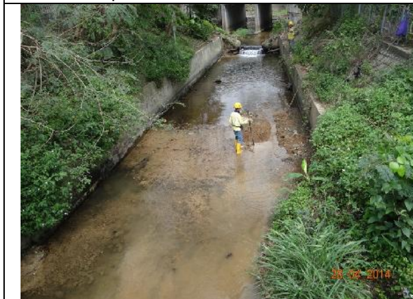
Photo 5 – The sand bags used to divide the river were removed and the worker removed the sediment washed away from the upper stream.
