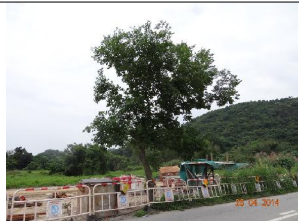
Photo 28 – The retained tree T025 was temporarily guyed to provide additional support to this tree.
