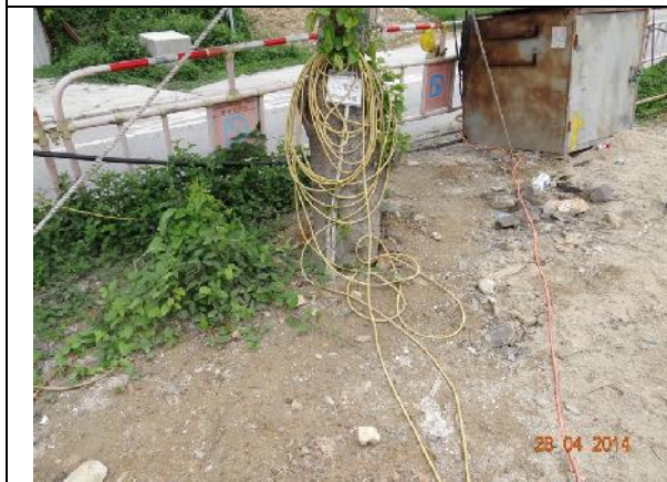
Photo 29 – Excessive soil were still piled close to the root flare of T025.
