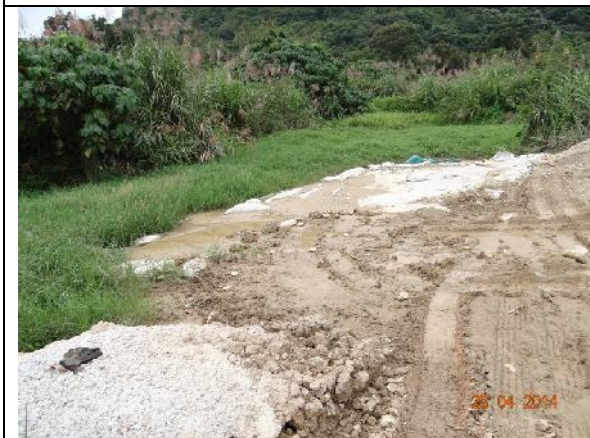
Photo 21 – Cement mortar along the southern boundary edge close to the wetland rehabilitation habitat was removed and the area was covered by a mat.
