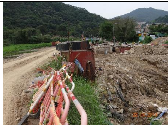
Photo 14 – A sedimentation tank was not in used.
