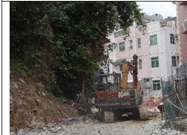
Photo 27 – Excavated soil and rocks and construction materials were noted piling close to the trunk base of the retained tree T103.
