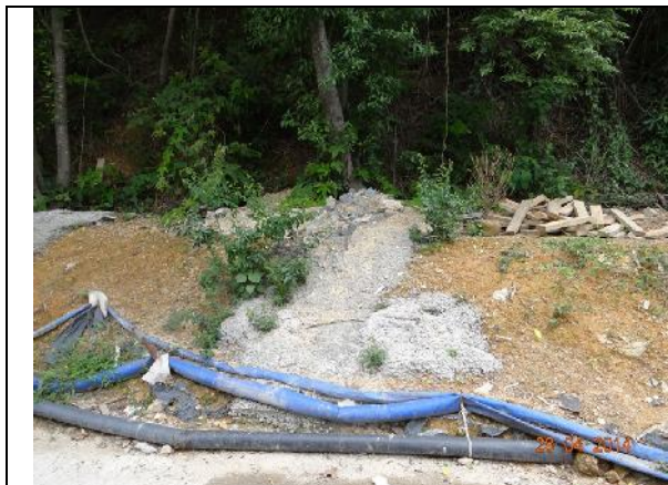
Photo 25 – Storage of construction materials and sand piling was noted close to the trunk flares and trunk of T093. Cement mortar was also noted on the soil surface close to T093.
