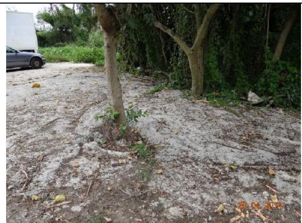
Photo 30 – Concrete pavement was observed close to the root flare of the tree group T089-091.
