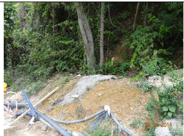
Photo 26 – Storage of construction materials and sand piling was noted close to the trunk flares and trunk of T094. Cement mortar was also noted on the soil surface close to T094.
