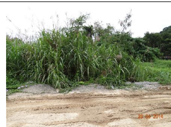
Photo 22 – Cement mortar was discharged next to the rehabilitation wetland near the exit point opposite to the tree group T021-029
