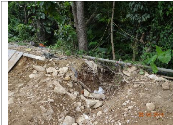
Photo 31 – Excavation work was noted between T153 and T155 and severe exposed roots were noted on these two trees.
