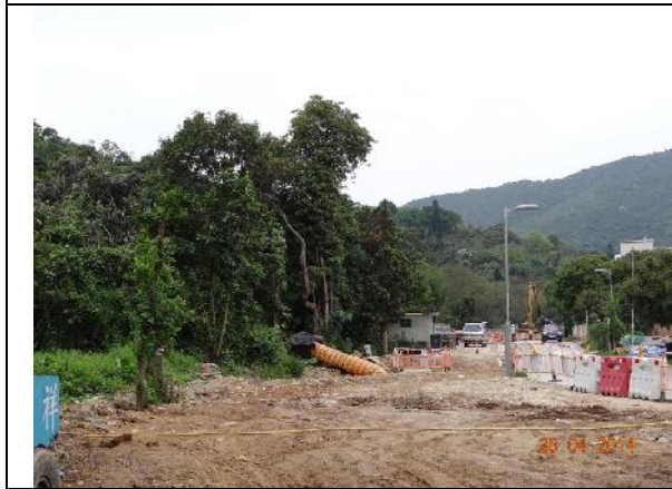
Photo 3 – Construction works for building the box culverts along Tung Tsz Road opposite to Wai Ha outside the public toilet.
