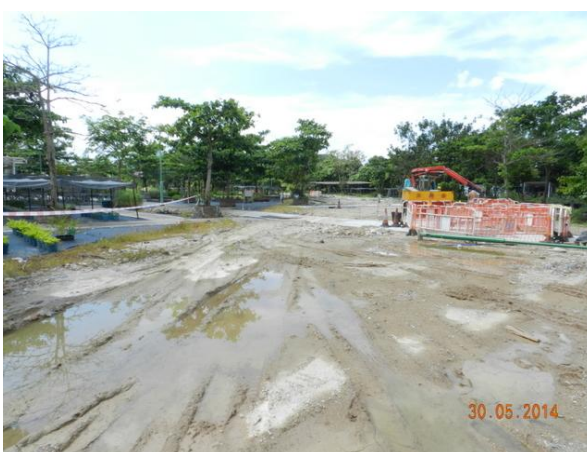
Photo 5 – The reinstatement work in Phase 2 area of Area B was demarcated by barrier tape, and no reinstatement work was in progress as observed in May 2014.
