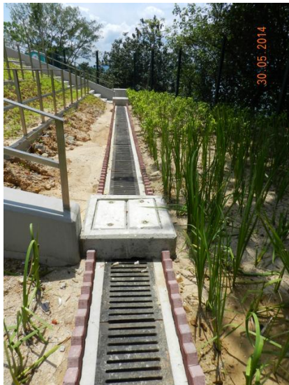
Photo 9 – The planting soil accumulated at the nearby planting area was found removed as observed on 30 th May 2014.
