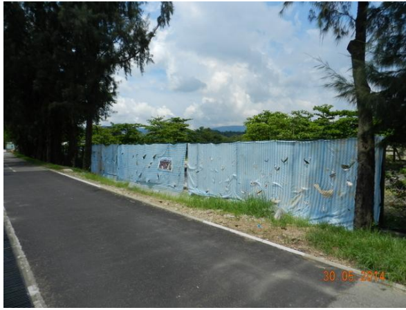
Photo 7 – Chain-link fence was reinstated at the eastern end of Phase 2 works area and covered by canvas sheets.
