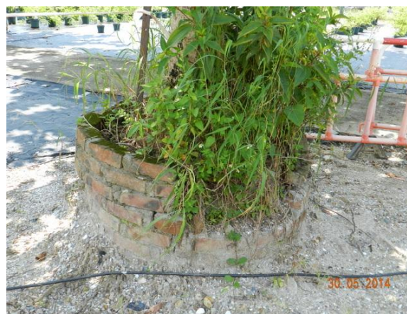
Photo 23 – The planter of U54 ( Terminalia catappa ) was broken and the exposed roots and soil was observed.
