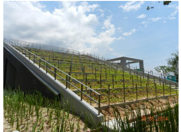
Photo 10 – The planted ground cover Arachis duranensis on the green roof was in fair condition.
