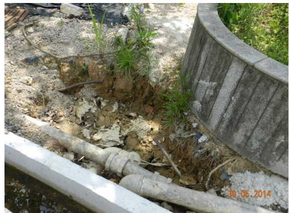
Photo 30 – The northern excavated area close to the planter of the retained tree A40 was not yet refilled.
