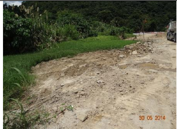
Photo 18 – Cement mortar along the southern boundary edge close to the wetland rehabilitation habitat was removed. The mat covering this area in mid-March 2014 was removed in May 2014.
