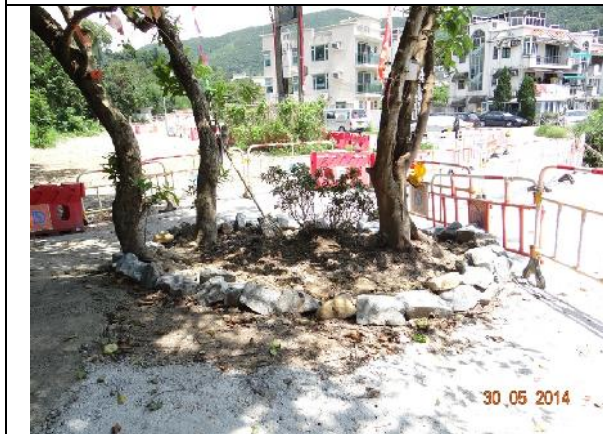
Photo 29 – Excavation work was noted very close to the tree group T181-T183. Excavated soil was noted piling around their trunk flare and the orange construction nets covered on the three trees were removed. These trees have been surrounded by some stones.
