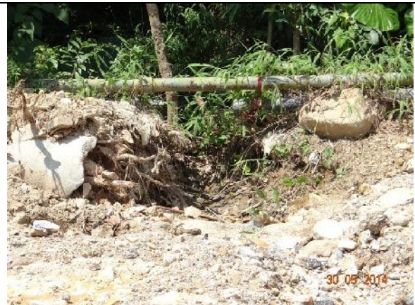
Photo 28 – Excavation work was noted between T153 and T155 and severe exposed roots were noted on these two trees.
