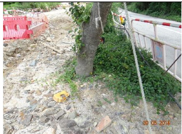
Photo 26 – Excessive soil were still piled close to the root flare of T025.
