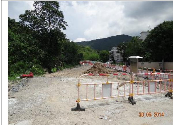
Photo 3 – Construction works for building the box culverts along Tung Tsz Road opposite to Wai Ha outside the public toilet.
