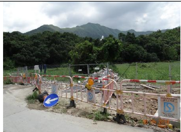
Photo 12 – A fenced area was seen on the field next to the construction site along the access to Treasure Spot Garden in March 2014. The area was still surrounded by chain-link fence by an unknown party.
