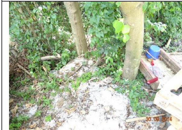
Photo 27 – Concrete pavement was observed close to the root flare of the tree group T089-091
