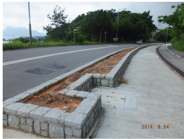
Photo 3 – The roadside planters along Ting Kok Road were constructed but no shrub planting has been carried out.
