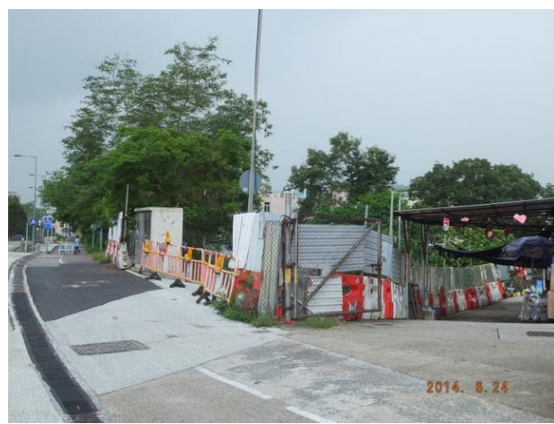
Photo 1 – Temporary construction hoardings have been established around the works area at Wai Ha River estuary and the work was completed.
