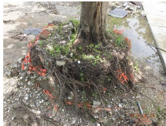
Photo 24 – The planter of another untagged Terminalia catappa next to U54 was broken, with exposed roots and soil.
