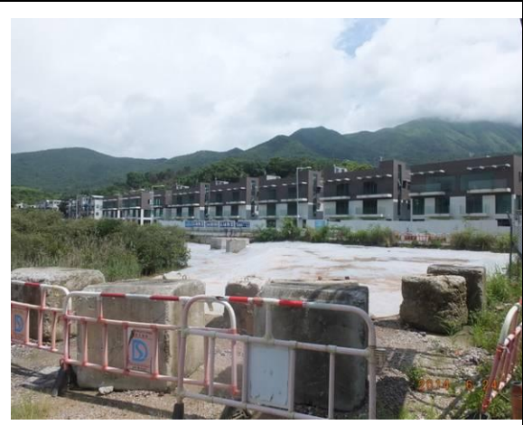
Photo 38 – The soil ground to the northwest of Tung Tsz Nursery has been hydroseeded.
