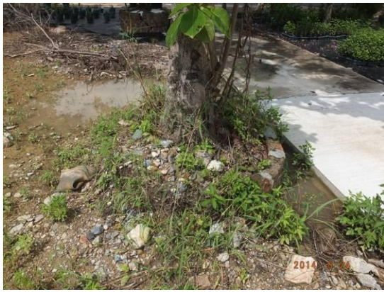
Photo 21 – Close-up view of the broken planter of U47.
