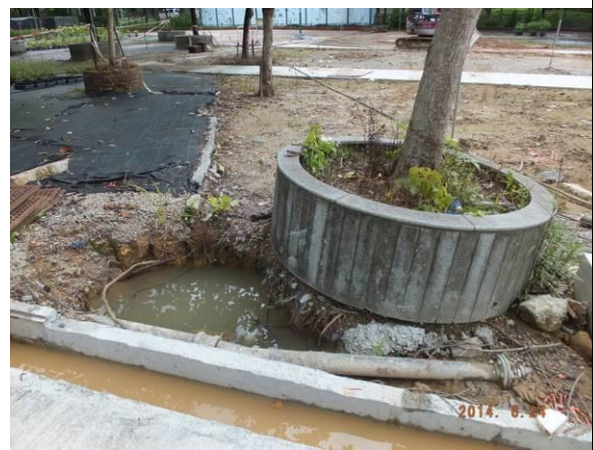
Photo 30 – The northern excavated area close to the planter of the retained tree A40 was not yet refilled.
