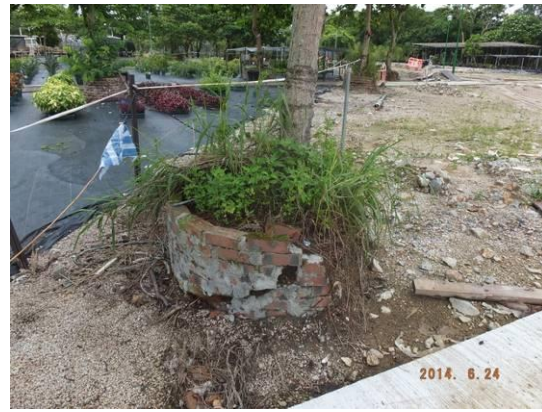
Photo 22 – The planter of an untagged Terminalia catappa next to U54 was broken, with exposed roots and soil.
