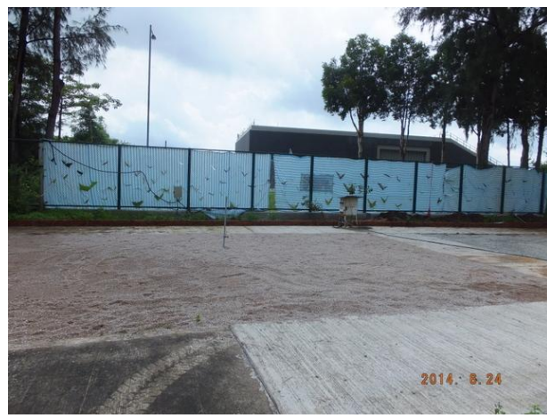
Photo 7 – Chain-link fence was reinstated at the eastern end of Phase 2 works area and covered by canvas sheets.
