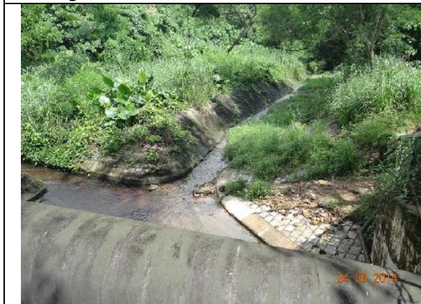
Photo 17 – No direct water discharge into the upper stream of Wai Ha River was observed as the construction works have been concentrated at the lower end of the river.
