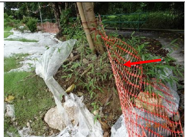
Photo 30 – Excavation work was noted next to an untagged tree ( Macaranga tanarius var. tomentosa ) (Red arrow). Severe exposed roots were noted on this tree.
