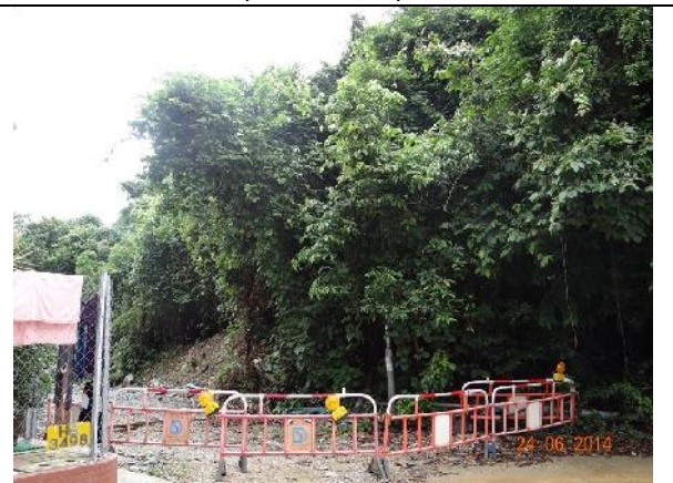
Photo 10 – Construction works have been stopped at the end of the Treasure Spot Garden II near the retained tree T103 and the works area was surrounded by temporary construction barriers and chain-link fence.
