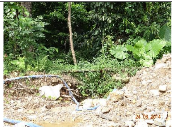
Photo 26 – Excavation work was noted between T153 and T155 and severe exposed roots were noted on these two trees.
