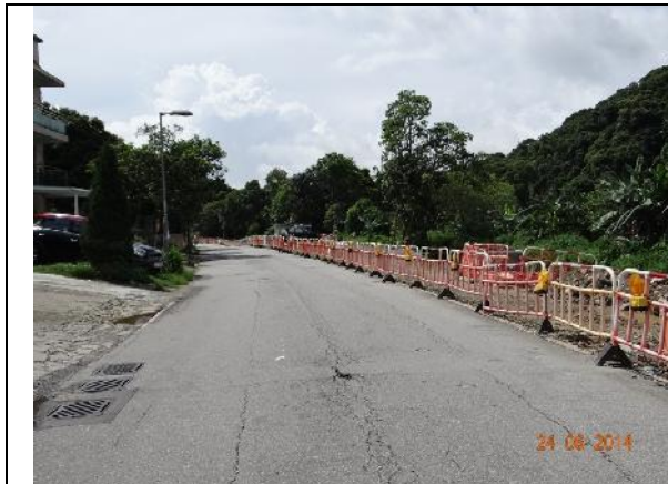
Photo 1 – Temporary hoardings have been erected along Tung Tsz Road opposite to Wai Ha.
