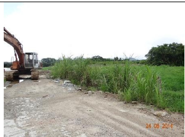
Photo 6 – Temporary construction barriers surrounding the eastern side of the wetland rehabilitation area were removed.
