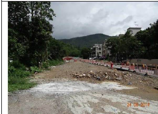
Photo 3 – Construction works for building the box culverts along Tung Tsz Road opposite to Wai Ha outside the public toilet have been stopped.
