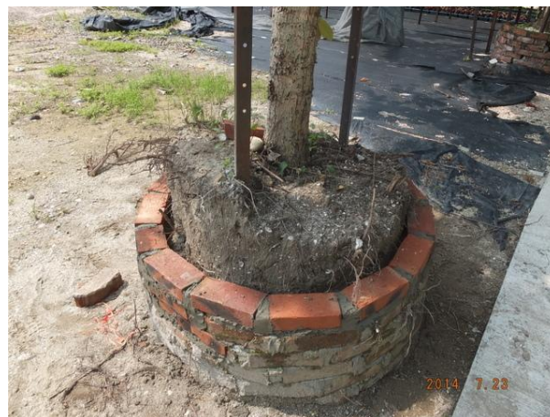
Photo 22 – The planter of U51 was repaired, but it was lower than the soil surface of the tree.
