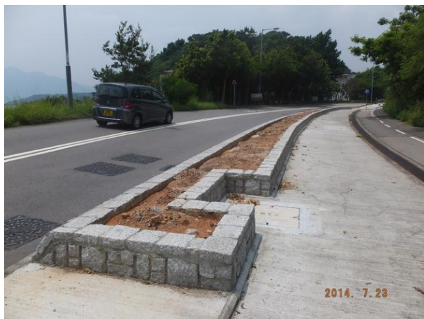
Photo 3 – The roadside planters along Ting Kok Road were constructed but no shrub planting has been carried out.
