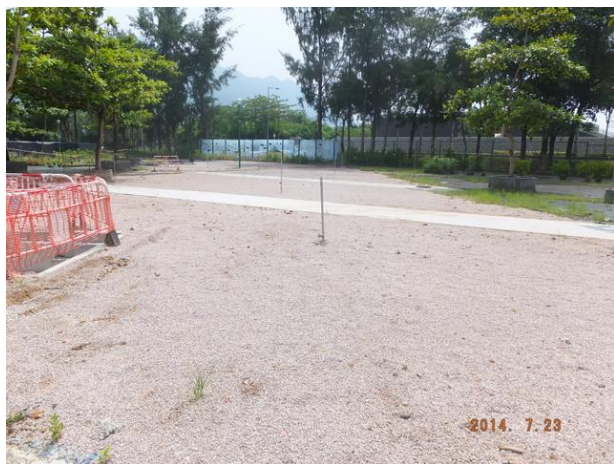
Photo 5 – The reinstatement work of the nursery in Phase 2 of Area B was almost completed.
