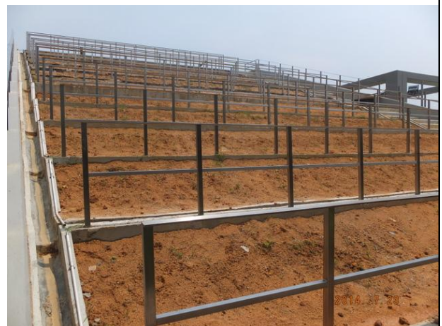
Photo 12 – The planted ground cover Arachis duranensis on the sloping green roof was removed.
