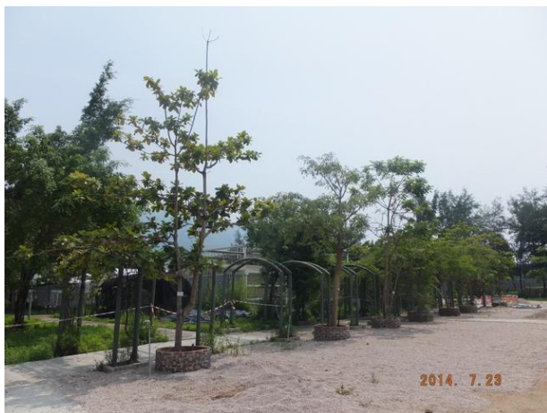
Photo 11 – Examples of other repaired planters of the relocated trees in Phase 1 works area.
