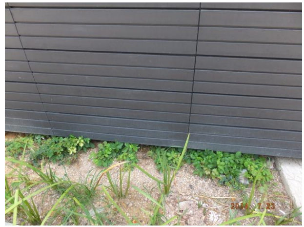
Photo 14 – Close-up view of the planted climber Parthenocissus dalzielii on the ground for vertical greening on the pump house.
