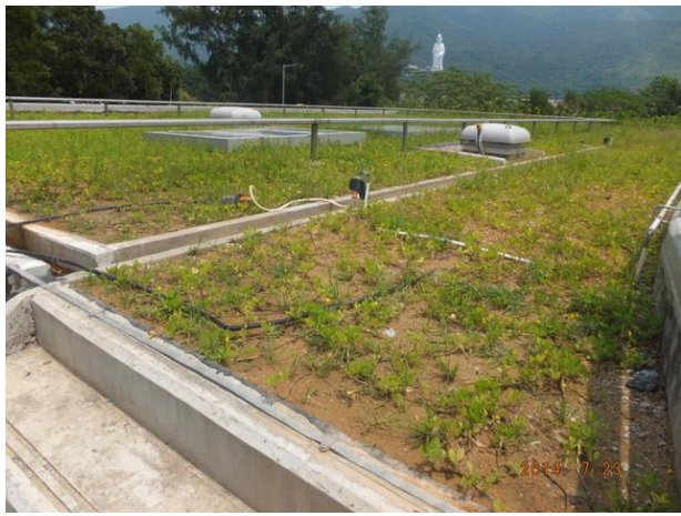
Photo 13 – The ground cover Arachis duranensis planted on the green roof was in fair condition.
