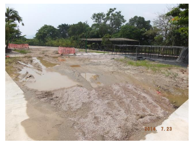
Photo 4 – The reinstatement work of the nursery ground in Phase 1 of Area B was under progress.
