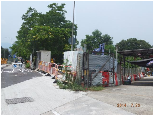
Photo 1 – Temporary construction hoardings have been established around the works area at Wai Ha River estuary. Minor rock breaking work was noted on 23 rd July 2014.
