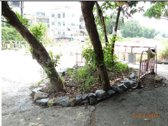
Photo 29 – Excavation work was noted very close to the tree group T181-T183. Excavated soil was noted piling around their trunk flares and the orange construction nets covering on the three trees were removed. These trees have been surrounded by some stones.
