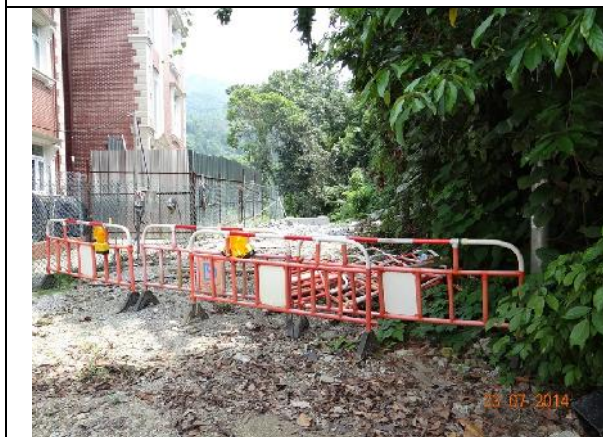
Photo 9 – Construction works have been stopped at the end of the Treasure Spot Garden II near the retained tree T103 and the works area was surrounded by temporary construction barriers and chain-link fence.
