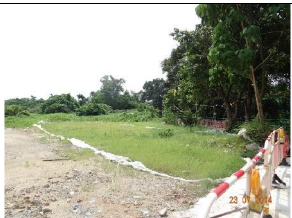
Photo 10 –The construction materials stored on the works area near the location of the previously removed tree T190 ( Ficus hispida ) were removed. This area has been covered by a mat in May 2014 and hydroseeding was applied in June 2014.
