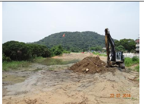
Photo 18 – Excavation works were carried out next to the wetland opposite to Jade View Villa during the site inspection on 23 rd July 2014. The area was waterlogged and unclear water overflowed into the nearby marsh area.
