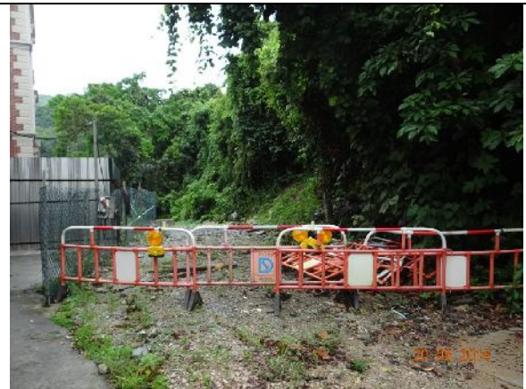
Photo 10 – Construction works have been stopped at the end of the Treasure Spot Garden II near the retained tree T103 and the works area was surrounded by temporary construction barriers and chain-link fence.
