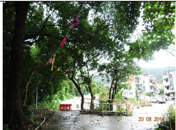
Photo 28 – Excavation work was noted very close to the tree group T181-T183 in May 2014. Excavated soil was noted piling around their trunk flares and the orange construction nets covering on the three trees were removed. These trees have been surrounded by some stones to demarcate the tree group area.
