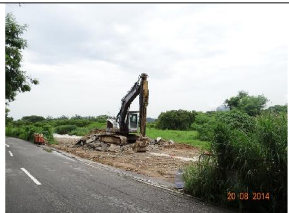
Photo 12 – An excavator was removing the cement mortar next to the exit point opposite to the tree group T021-029 ( Leucaena leucocephala ) as observed on 20 th August 2014.
