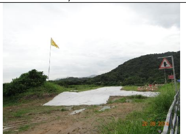
Photo 6 – Construction works next to the wetland opposite to Jade View Villa have been stopped. The site was covered by a mat.
