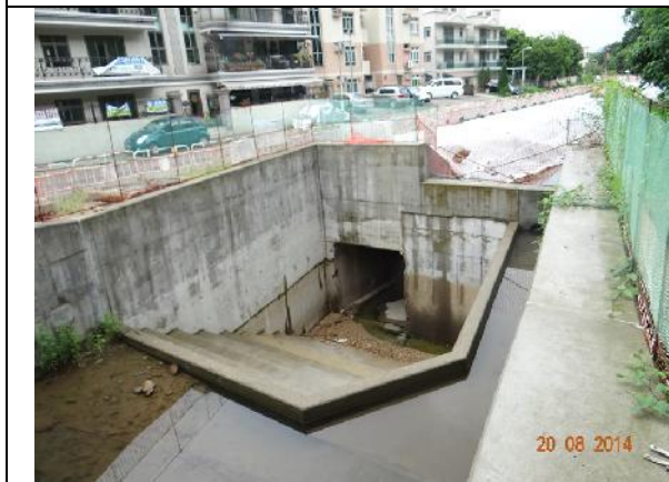
Photo 3 – Construction works have been stopped next to Wai Ha River.
