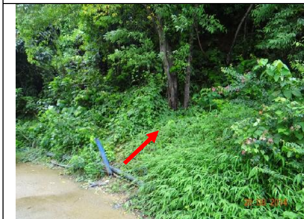
Photo 21 – Storage of construction materials and sand piling close to the trunk flare of T094 was removed. However, cement mortar has been noted on the soil surface close to T094. This area was covered by ground vegetation as observed in August 2014 (indicated by Red arrow).
