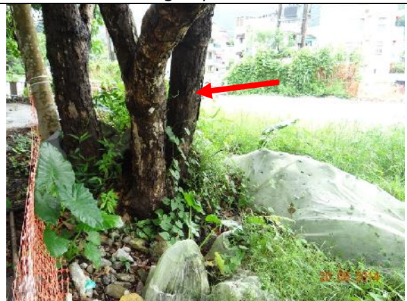
Photo 30 – Excavation work was noted next to an untagged tree ( Cleistocalyx nervosum ) (Red arrow). Severe exposed roots were noted on this tree.
