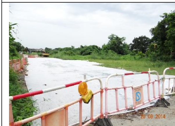
Photo 5 - Construction works next to the wetland near the location of the previously removed tree T190 have been stopped. The site was covered by a mat.
