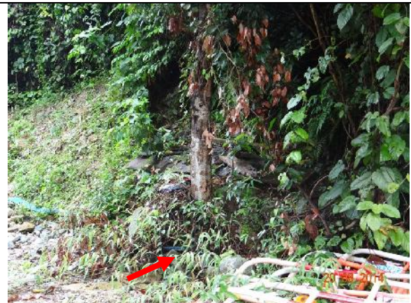
Photo 24 – Excavated soil and rocks, and construction materials were still noted piling close to the trunk base of the retained tree T103.
