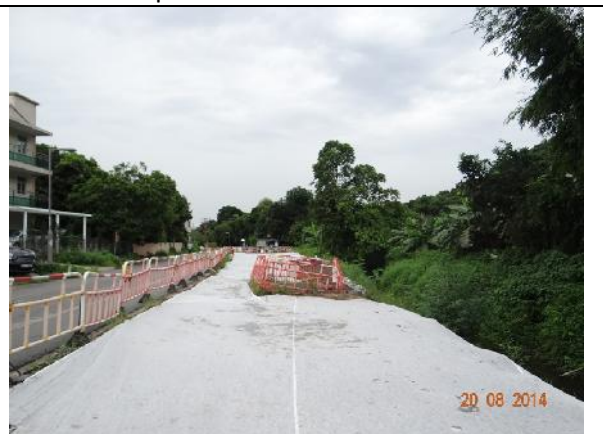
Photo 4 – Construction works for building the box culverts along Tung Tsz Road opposite to Wai Ha outside the public toilet have been stopped. The site was covered by a mat.
