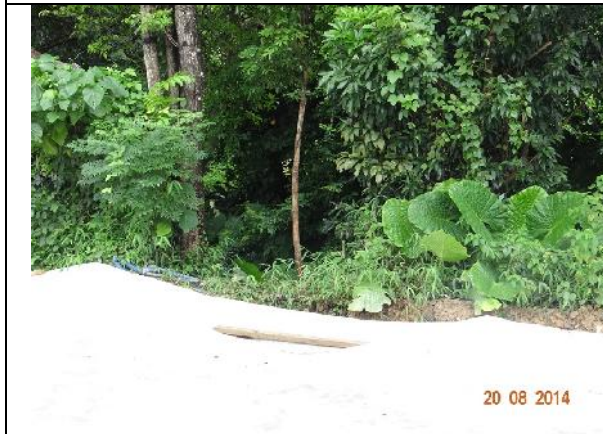
Photo 27 – Excavation work was noted between T153 and T155, and severe exposed roots were noted on these two trees.
