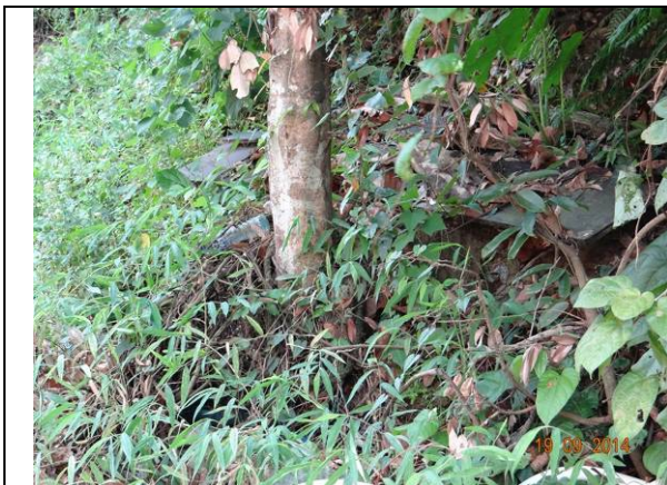
Photo 25 – Excavated soil and rocks, and construction materials were still noted piling close to the trunk base of the retained tree T103.
