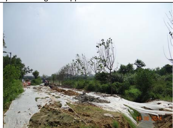
Photo 6 - Planting of the compensatory trees was in progress on 19 th September 2014 opposite to the tree groups T030-033 and T035-036.
