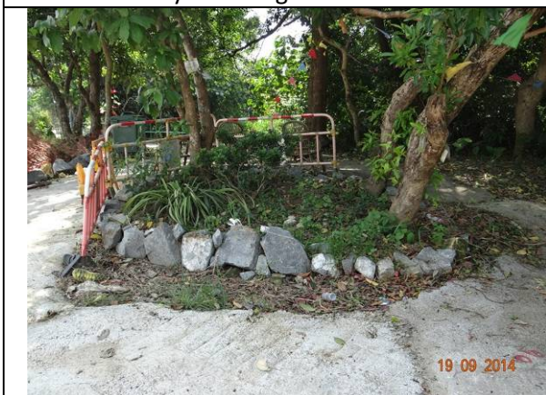
Photo 29 – Excavation work was noted very close to the tree group T181-T183 in May 2014. Excavated soil was noted piling around their trunk flares and the orange construction nets covering on the three trees were removed. These trees have been surrounded by some stones to demarcate the tree group area by the villagers.
