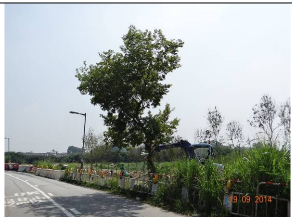
Photo 26 – The retained tree T025 was temporarily guyed to provide additional support to this tree.
