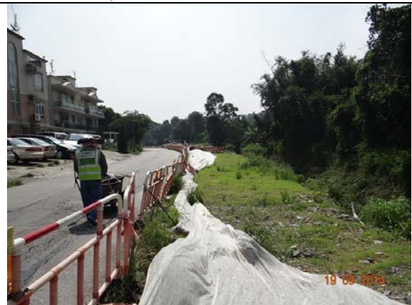
Photo 4 – Construction works for building the box culverts along Tung Tsz Road opposite to Wai Ha outside the public toilet have been stopped. Hydroseeding was applied on the site.
