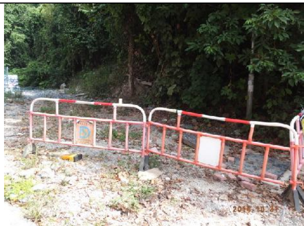
Photo 11 – Construction works have been stopped at the end of the Treasure Spot Garden II near the retained tree T103 and it was surrounded by temporary construction barriers.
