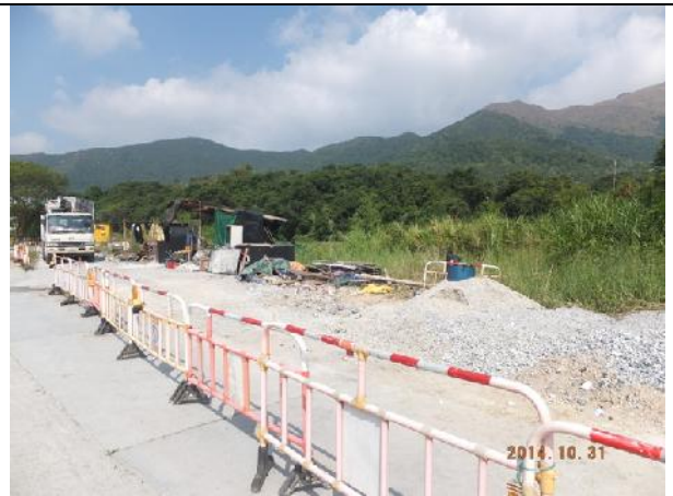
Photo 2 – Temporary hoardings have been erected along the access road from Tung Tsz Road to Treasure Spot Garden II.
