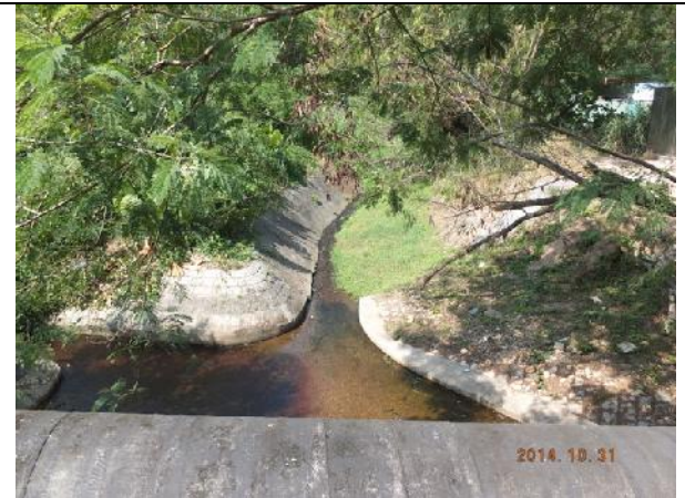
Photo 16 – No direct water discharge into the upper stream of Wai Ha River was observed as all major construction works were completed.
