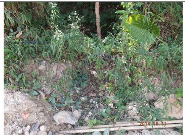
Photo 26 – Excavation work was noted previously between T153 and T155 in April 2014, and exposed roots were noted on these two trees. Surrounding ground was covered by vegetation.
