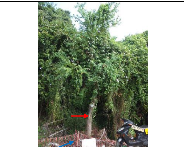
Photo 10 – The untagged tree (indicated by Red arrow) was guyed at the edge of the parking area within a Tree Protection Zone demarcated by orange construction nets (indicated by Blue arrow).
