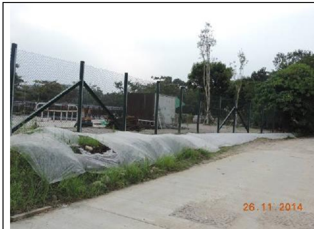
Photo 7 – Main entrance of Phase 1 construction work area was reinstated with chain-link fence and the nearby area was hydroseeded.
