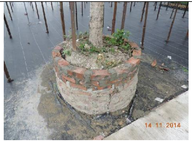
Photo 20 – The planter of U51 was repaired and built up to the soil surface of the tree.
