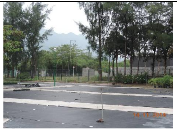
Photo 6 – Chain-link fence was reinstated at the eastern end of Phase 2 works area and the canvas sheet previously found on the fence was removed.
