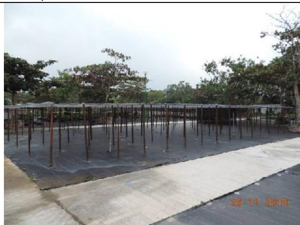
Photo 5 – The reinstatement work of the nursery in Phase 1 of Area B was under progress and almost completed.
