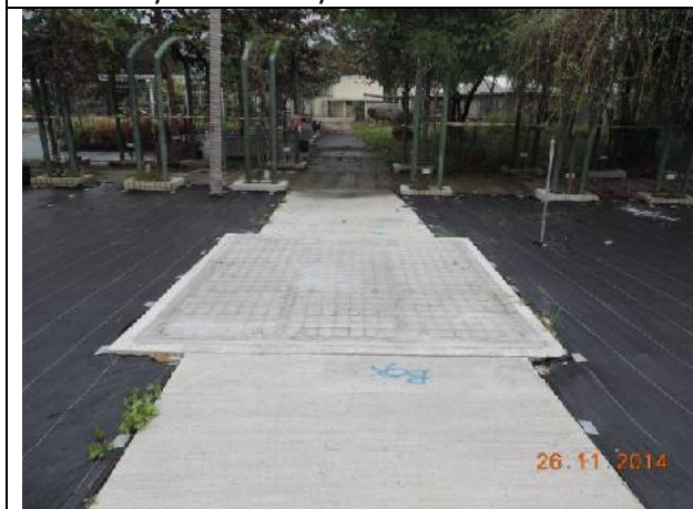
Photo 9 –The manhole was closed and the temporary construction hoardings surrounding the manholes were removed.
