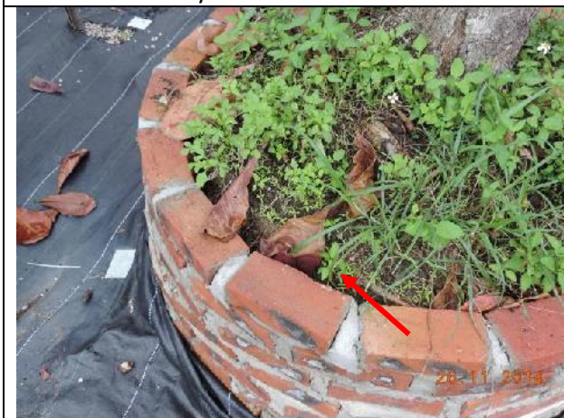
Photo 21 – Example of gap between the root ball and the inner surface of the new planter.
