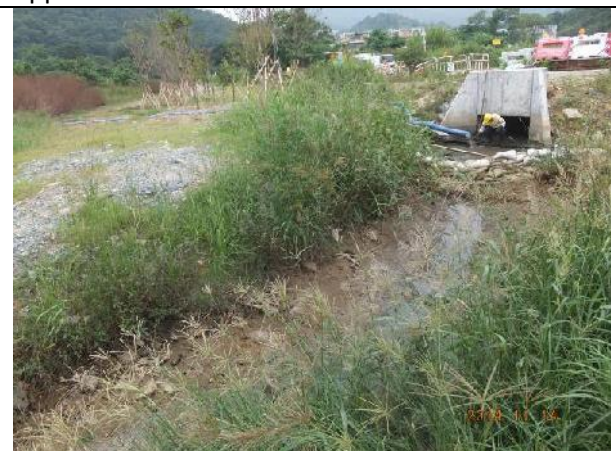
Photo 18 – Water used to clean the underground box culvert was discharged through the drainage outfall to the tidal marsh area.
