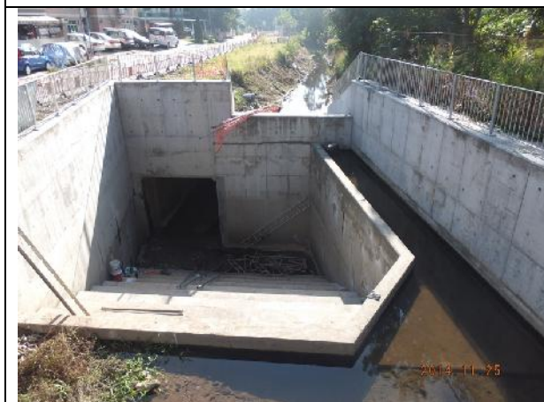
Photo 3 – No active construction works was carried out in the built box culvert and its associated structure.
