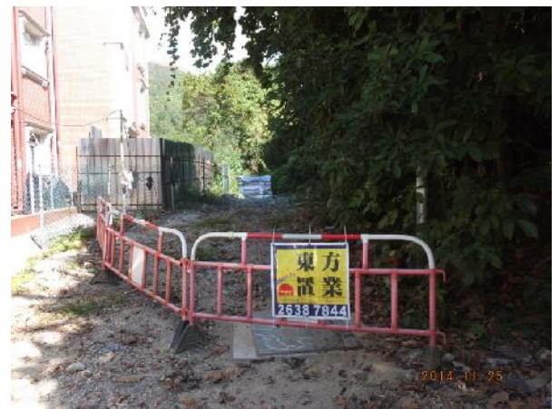
Photo 12 – Construction works have been stopped at the end of the Treasure Spot Garden II near the retained tree T103 and it was surrounded by temporary construction barriers.
