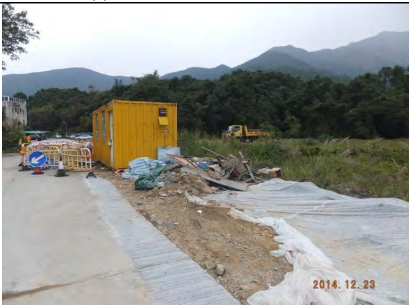
Photo 6 – Minor civil work was continued along the access path leading from Tung Tsz Road to Treasure Spot Garden II.
