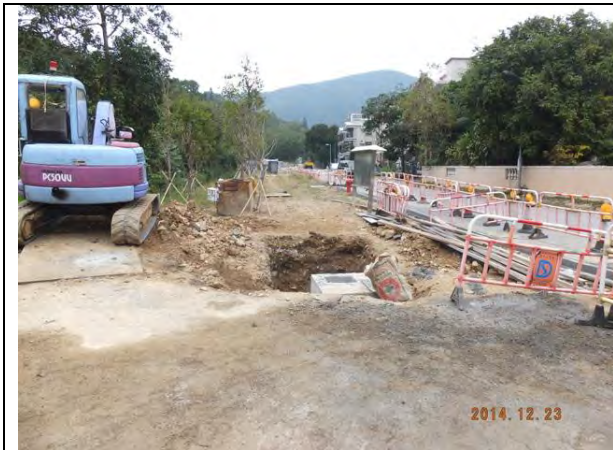
Photo 7 – Minor civil work was conducted for building a refuse collection point opposite to Wai Ha area.
