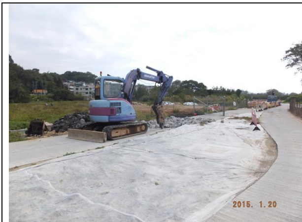
Photo 7 – Minor civil work was conducted on the temporary access road in Treasure Spot Garden II.
