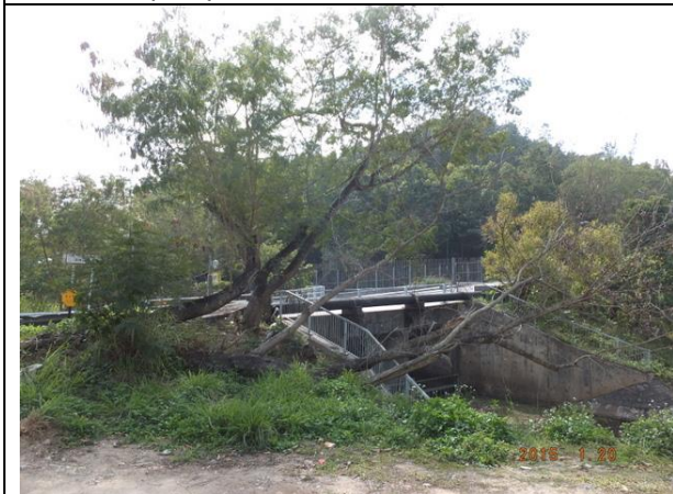
Photo 29 – The tree trunk from the tree group of T085-T087 at the junction of Tung Tsz Road and Tung Tsz Shan Road was partly uprooted and significantly leaned towards Wai Ha River.
