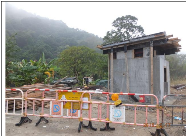
Photo 7 – Minor civil work was still carried out in the works area opposite to Wai Ha.
