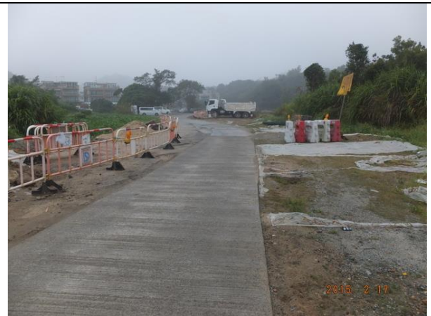
Photo 8 – Minor civil work was conducted on the temporary access road in Treasure Spot Garden II.
