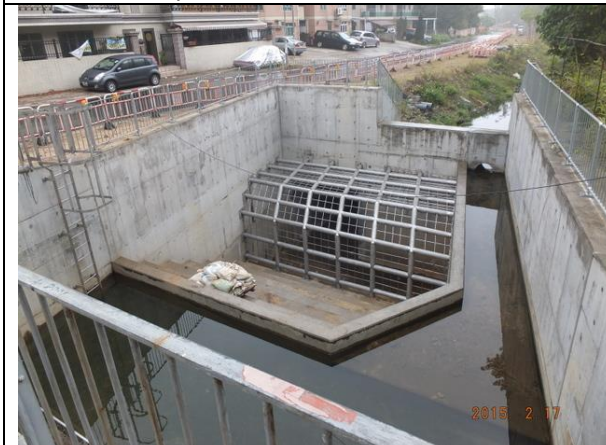
Photo 5 –The box culvert and the associated drainage work were completed at the upper part of Wai Ha River.
