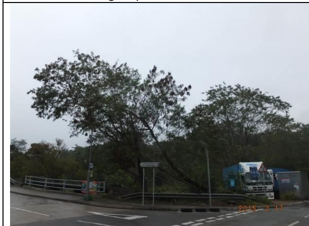
Photo 29 – The tree trunk from the tree group of T085-T087 at the junction of Tung Tsz Road and Tung Tsz Shan Road was partly uprooted and significantly leaned towards Wai Ha River.
