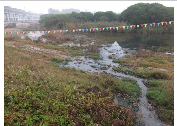
Photo 4 – Construction works opposite to San Tau Kok was already completed and fully vegetated.
