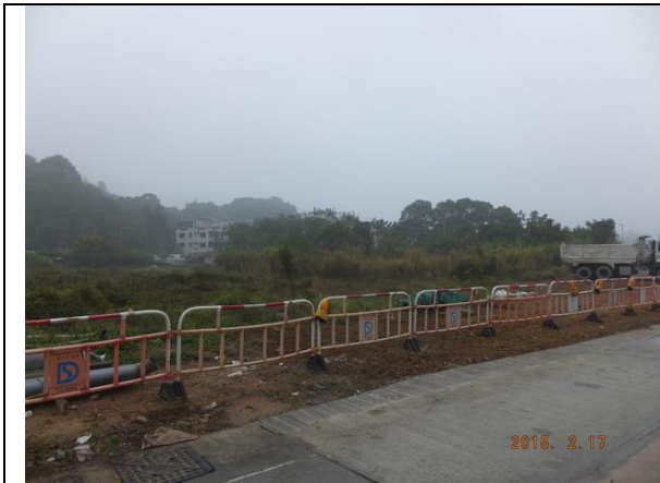
Photo 1 – Temporary hoardings were erected again along part of the access path towards Treasure Spot Garden II.
