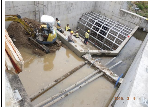
Photo 15 – Minor dredging work was carried out to remove the mud at the desilting part of the intake structure near the Wai Ha River.
