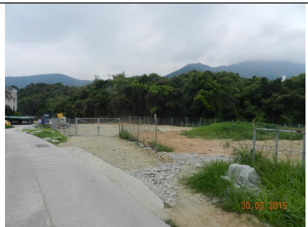
Photo B14 - A fenced area, which was erected by the villagers, has been recorded next to the works area of this Project.
