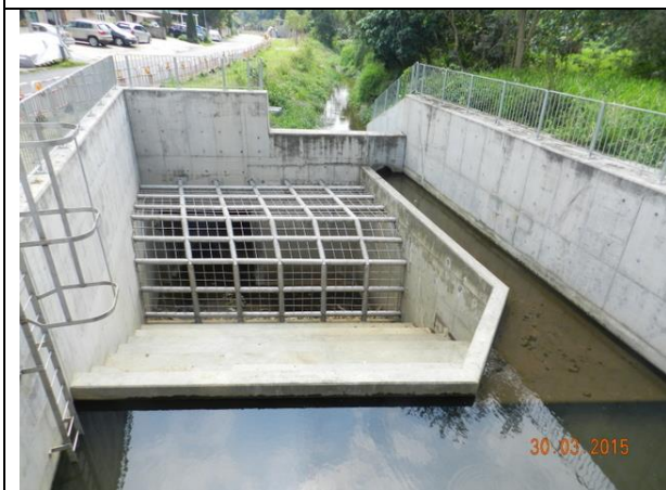
Photo B5 –The box culvert and the associated drainage work were completed at the upper part of Wai Ha River.
