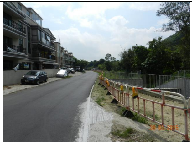
Photo B2 – Temporary hoardings erected along Tung Tsz Road and opposite to Wai Ha.
