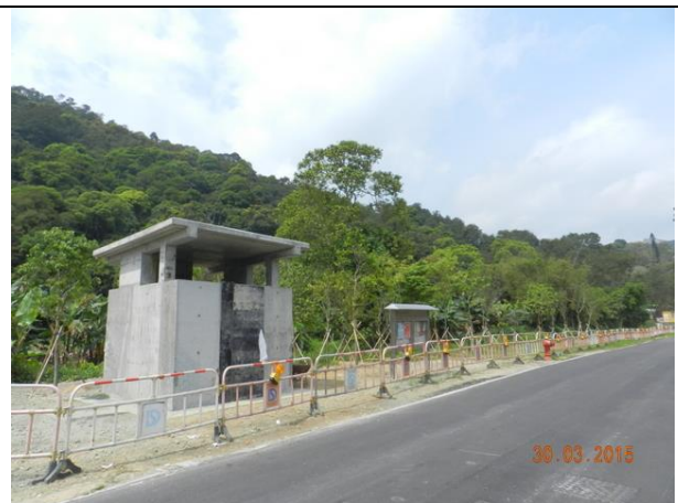
Photo B8 – The minor civil work opposite to Wai Ha area was completed by end of March 2015.
