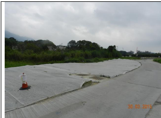
Photo B7 – The work along the access road in Treasure Spot Garden II was completed and the area was hydroseeded.
