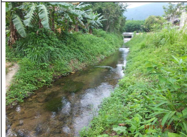
Photo B17 – Both bunds along Wai Ha River were naturally vegetated.
