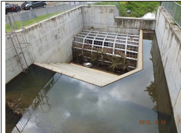
Photo B13 – The box culvert and the associated drainage work were completed at the upper part of Wai Ha River.
