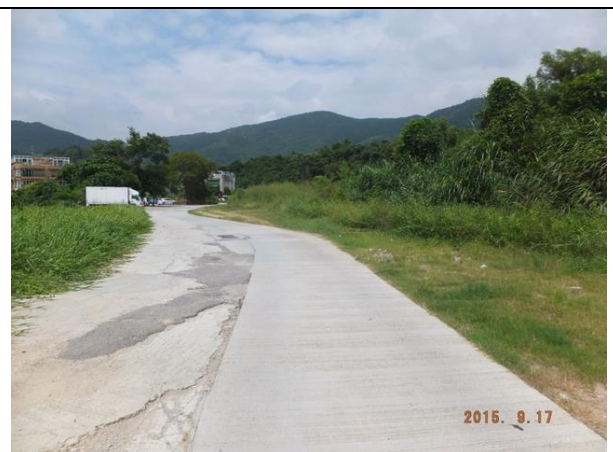
Photo B10 – The reinstated area above the drain pipe along the access path leading towards Treasure Spot Garden II.
