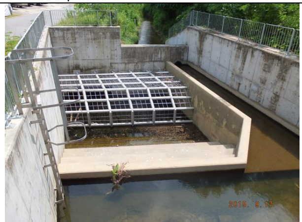
Photo B12 – The box culvert and the associated drainage work were completed at the upper part of Wai Ha River.
