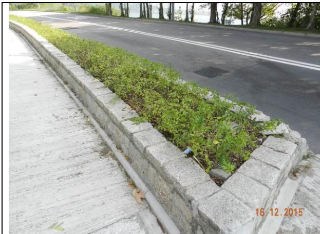
Photo A1 – Planters at Ting Kok Road were hydroseeded and planted with shrubs.
