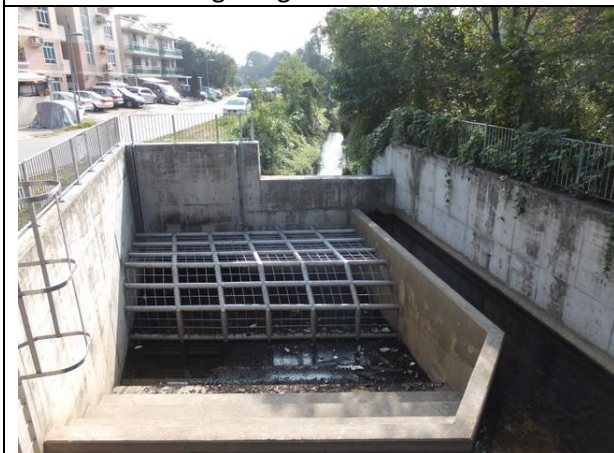
Photo B9 – The box culvert and the associated drainage work were completed at the upper part of Wai Ha River.
