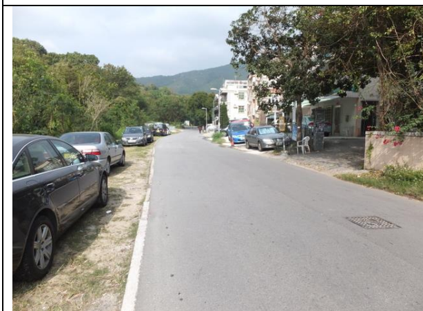
Photo B11 – The original Tung Tsz Road in Wai Ha area was reinstated.
