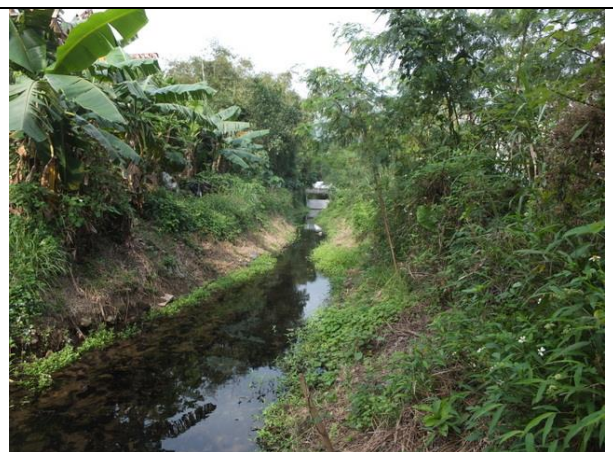
Photo B12 – Both stream banks of Wai Ha River were reinstated and naturally vegetated with self-seeded plants.
