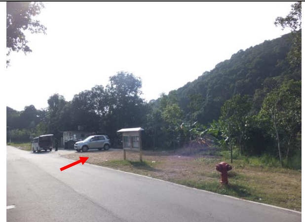
Photo B14 – The new refuse collection chamber (location indicated in red arrow) built in area opposite to Wai Ha was found being demolished.
