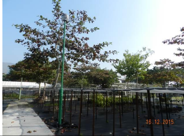
Photo A7 – Example of the completed reinstatement works within the nursery (such as lamp posts, shelters for potted plants and new planters for the transplanted tree).
