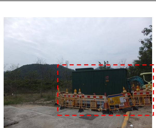
Photo B6 – Previous excavation work related to CLP Project was carried out at the locations where the five missing compensatory trees were planted. No tree replacement was noted.
