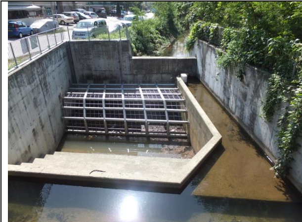
Photo 19 – The box culvert and the associated drainage work were completed at the upper part of Wai Ha River.
