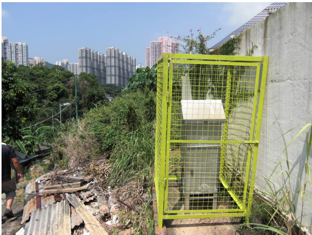
Ground floor boundary wall of house 51D of Wo Hop Shek San Tsuen
