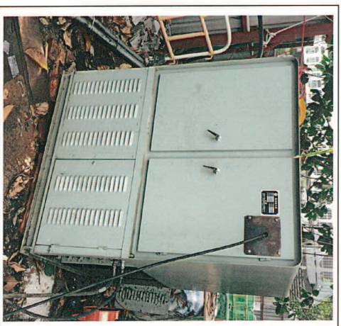
Power pack (diesel) 油渣動力供應器
