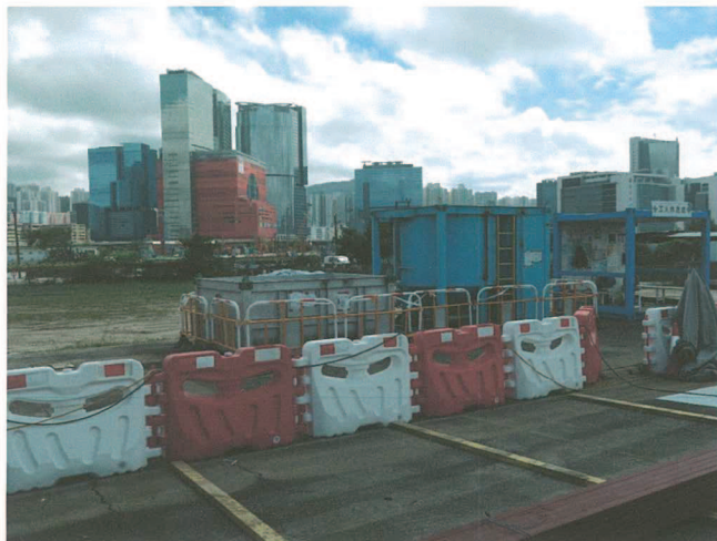
Wastewater Treatment Facility 廢水處理設施
